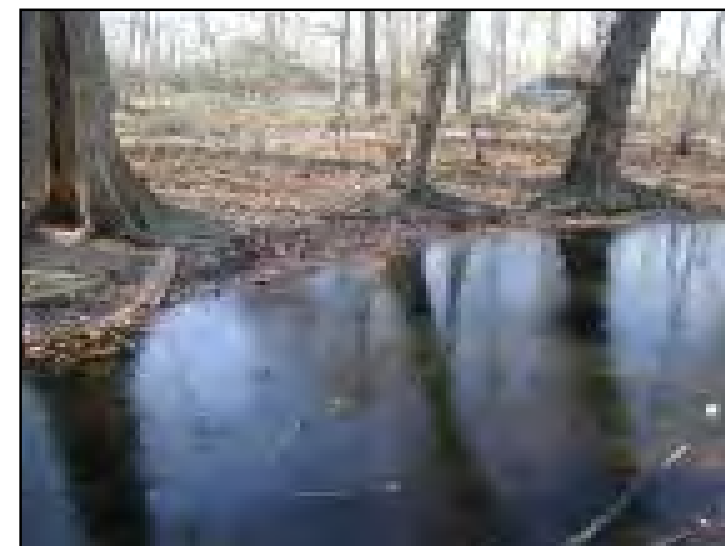
Example of minor erosion.
