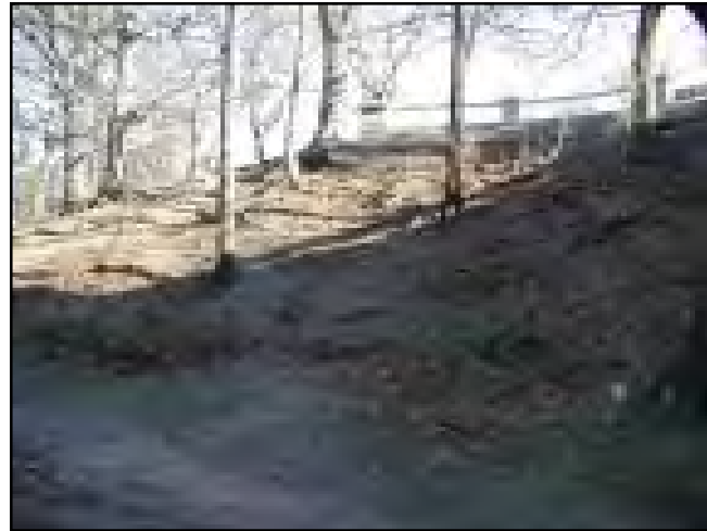
Example of major erosion.
