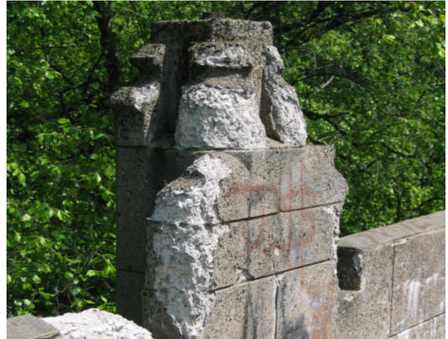
Photo 339 The top of this pier has severely spalled; note the top of the wall has been patched with a thin layer of mortar.
