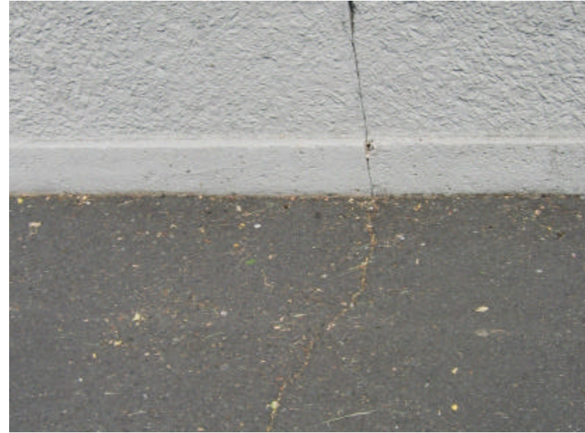
Photo 359 This crack continues from the parapet wall to the sidewalk.
