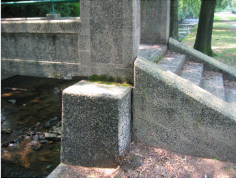
Photo 409 Spalling and organic growth at the base of the bridge's deck directly below the post at the north end of the bridge.
