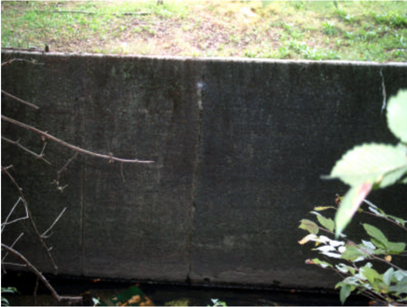
Photo 470 Detail of full-height, thru-wall crack at the south revetment east of Franklin Avenue.
