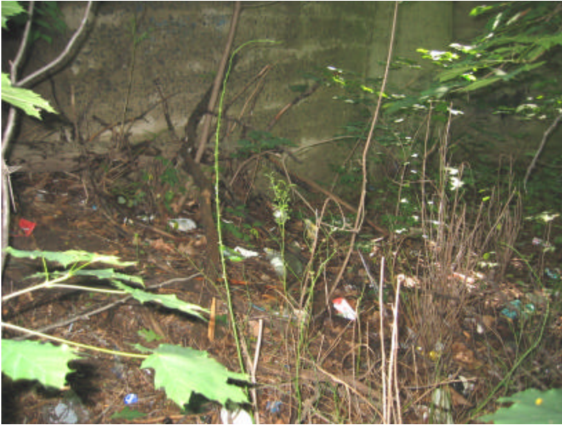
Photo 369 Embankments on the northwest side of the bridge; note the weeds and debris that are typical on all sides of the bridge.
