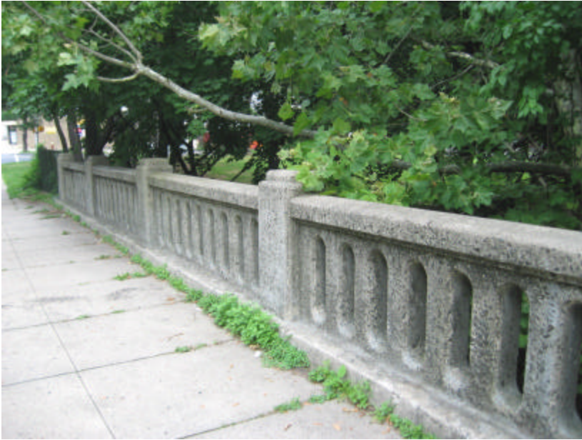
Photo 367 The east parapet railing; note that it is in good condition overall but does have some areas of severe spalling and cracking.
