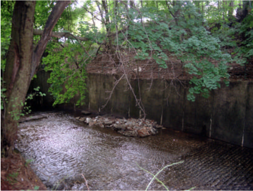
Photo 480 View of south embankment immediately west of the Mt. Prospect Avenue Bridge showing built-up debris in the paved channel; note that this section of wall is the only one at which salt deposits penetrate the wall construction.
