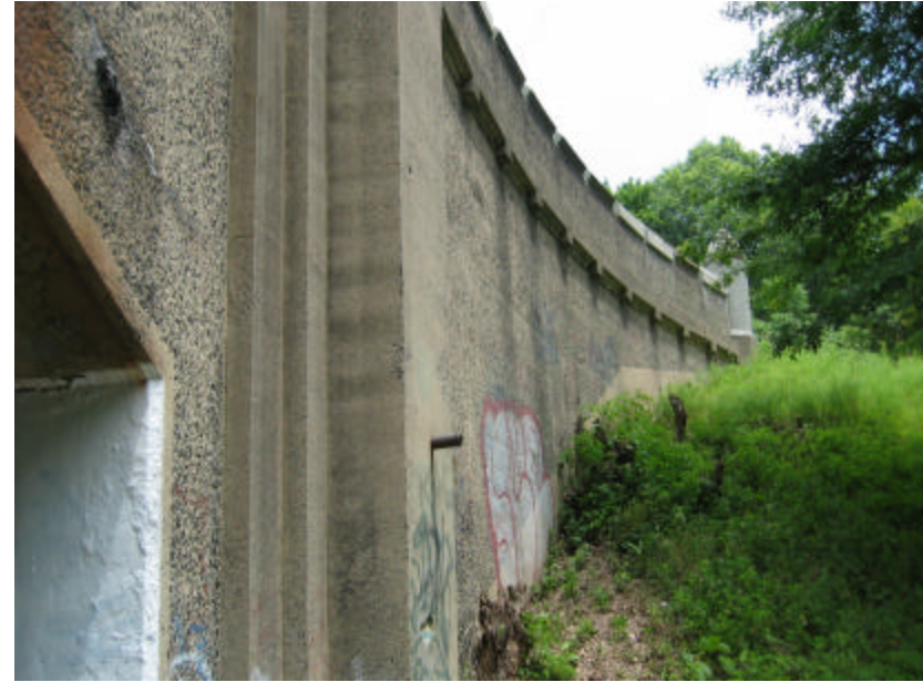
Photo 349 From the path that goes under the bridge, the arc of the wing wall is visible on the north side of the bridge; note that the buttress dividing the cheek and wing wall.
