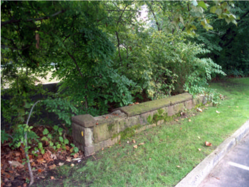
Photo 468 Detail of the stone wall at the culvert opening near Hendricks Field Golf Course on the north side of the channel; note that it is the only stone structure (other than bridges) than along the channel.
