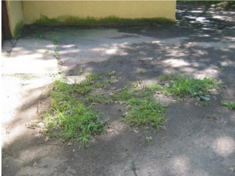
Photo 435 An area of paving in front of the garage door; note that this section is cracked, buckled and covered with grass and weeds.
