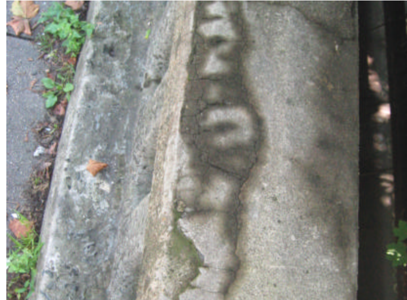
Photo 372 View looking down at cracking and spalling concrete on top of the railing; note that the cracks have absorbed a significant amount of moisture.
