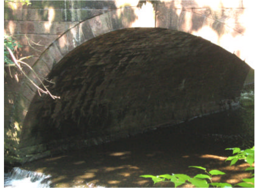
Photo 403 Visible staining and soiling of the archway caused by organic growth and efflorescence from water penetration.
