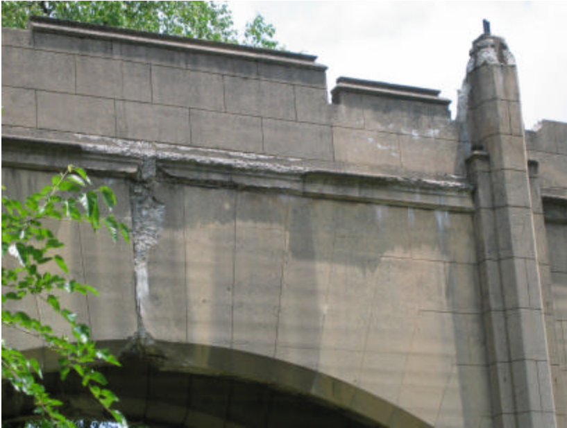
Photo 346 Spalling and cracking on the side of the bridge. The severe spalling continues from the underside of the bridge through the cheek wall and along the stringcourse.
