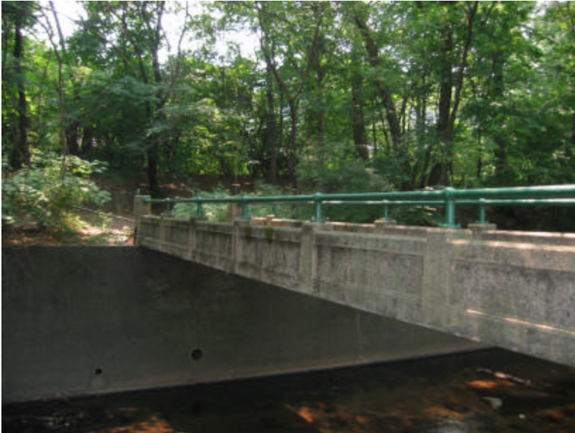
Photo 407 View southwest over the footbridge; note the organic growth and staining on the surface of the bridge.
