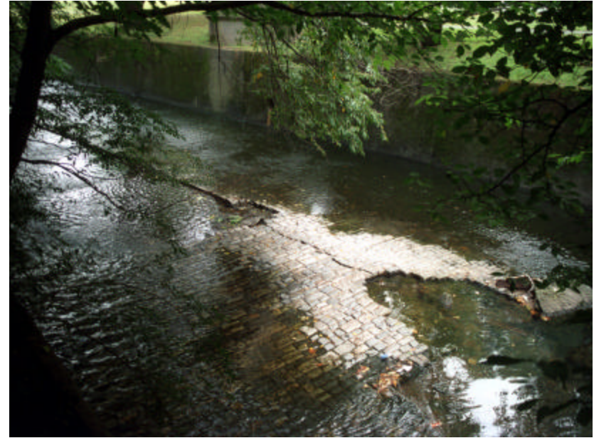
Photo 473 Detail of the channel bed west of the North Branch Brook Drive Bridge showing destroyed sections and the failure of the adjacent downstream bed (to the east).
