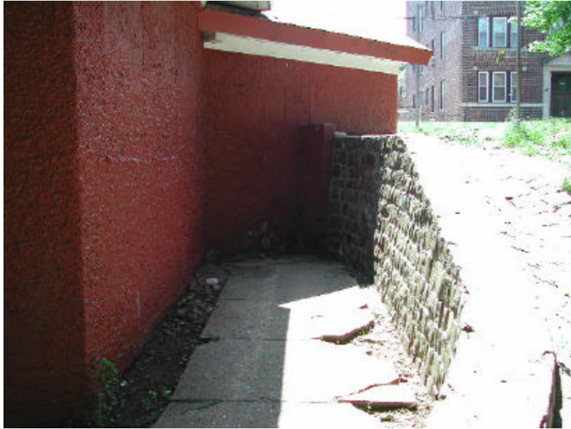
Photo 452 Detail of stone retaining wall, granite-paved gutter and poor-condition concrete paving.
