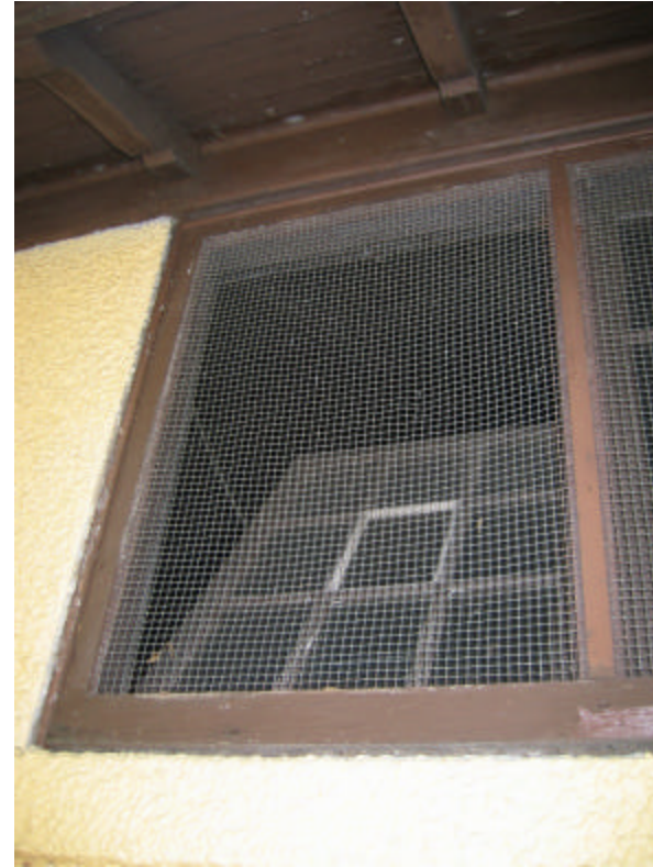
Photo 448 One of the original hopper windows in the open position; note the heavy metal screen covering the window opening.
