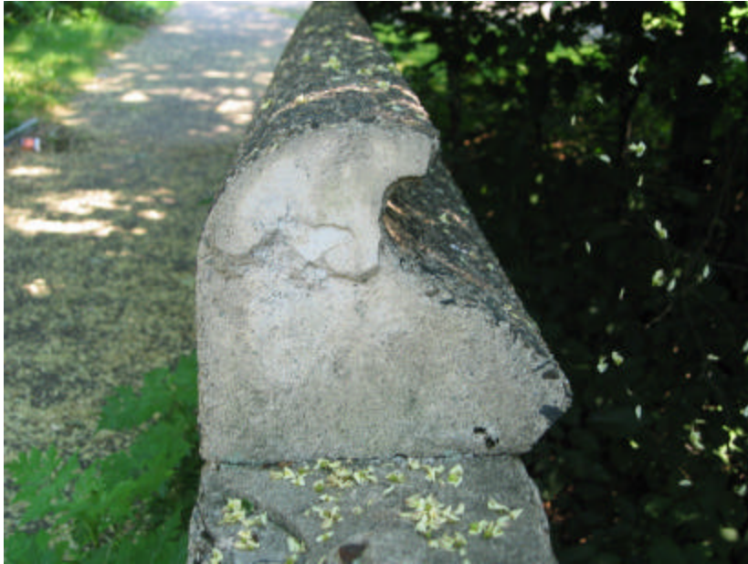
Photo 336 An original piece of coping on top of the parapet wall; note the detailed design.
