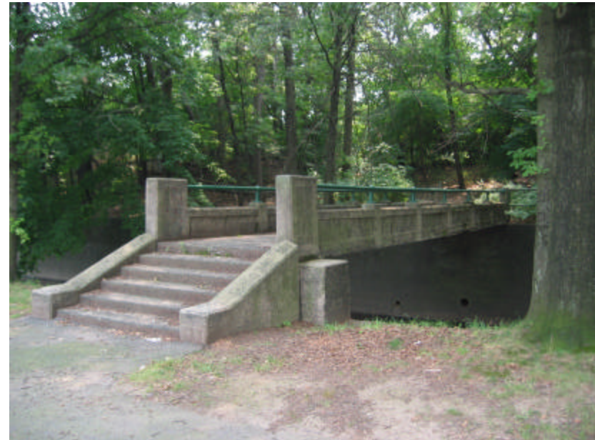
Photo 404 View south towards the footbridge; note the bare dirt around the site.
