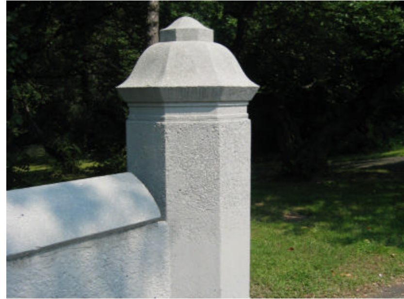
Photo 351 One of the posts that terminate the parapet wall; note that this post is in good condition and has been painted along with the wall.
