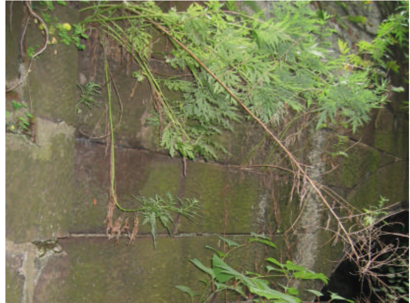
Photo 386 Plants and green organic growth covering brownstone surfaces on the west side of the bridge; note the open and exposed horizontal mortar joints.
