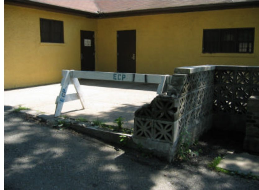
Photo 421 Area of the damaged concrete block wall west of the building.
