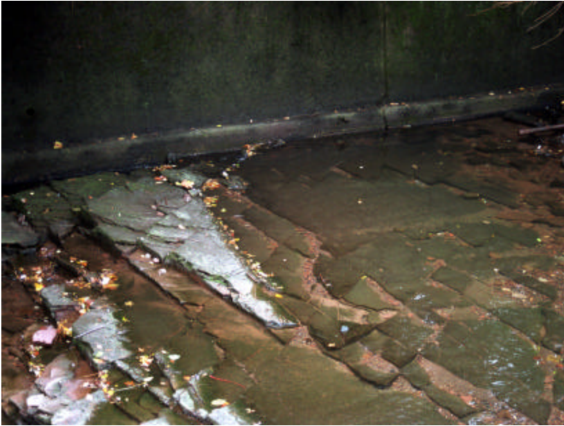
Photo 486 Detail of the south embankment east of the Summer Avenue Bridge; note that the concrete footing is exposed in this area.
