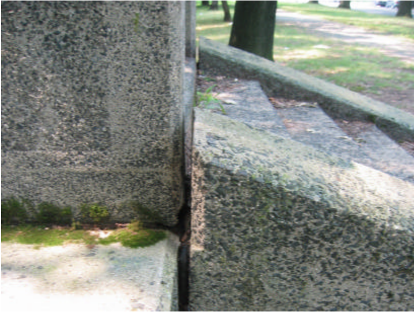
Photo 413 Open and exposed joints at the north end of the bridge.
