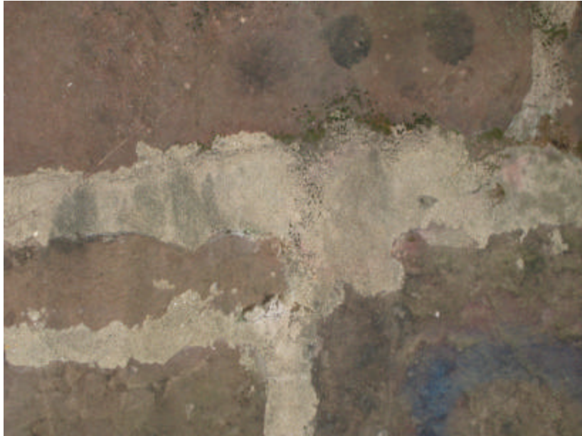
Photo 387 Substantially widened mortar joints caused by remedial patching of masonry on the west cheek wall.
