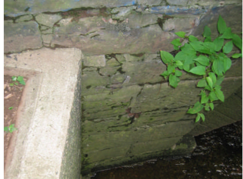
Photo 392 Looking down from the river bank towards the northeast wing wall, retaining wall and the river; note the open and exposed joints.
