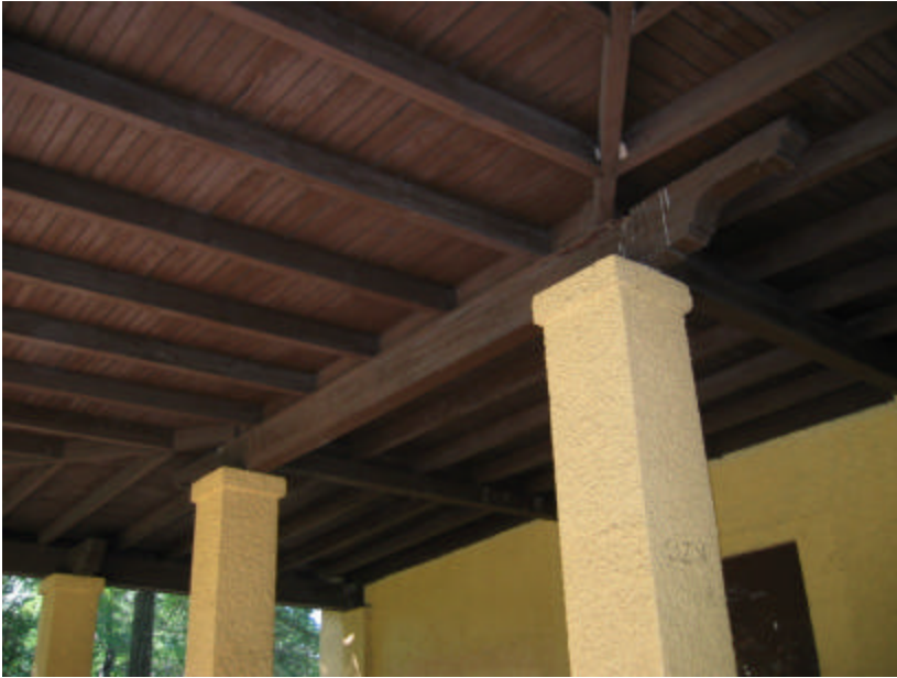
Photo 441 The rafters and beaded board sheathing; note that the beam is rotted above the right column.
