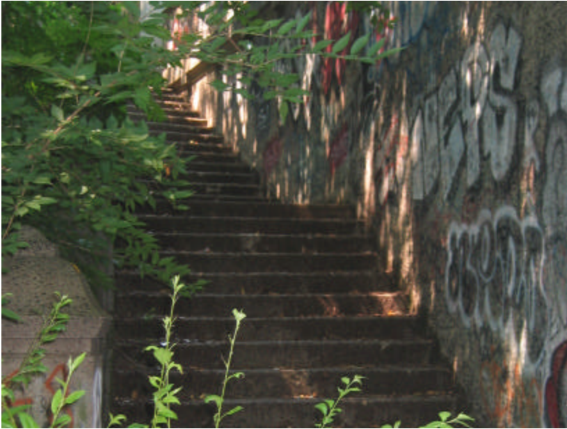
Photo 348 The staircase leading from a path along the Second River to the top of the bridge; note the graffiti on the wall.
