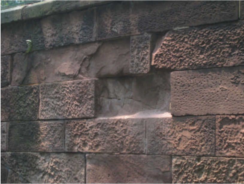
Photo 399 Severely spalling and delaminating brownstone; note that the once well-dressed surface is now weathered and worn.
