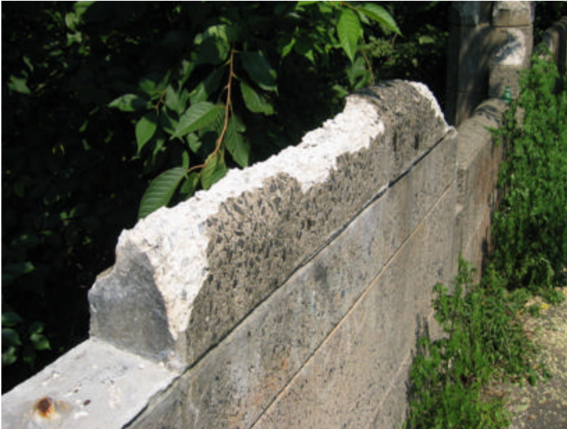
Photo 340 Significant spalling of the concrete coping caused by water absorption and the adverse effects of freeze-thaw cycles.
