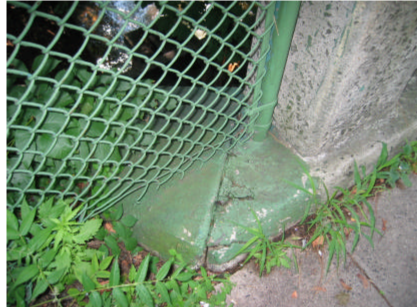
Photo 380 Chain link fence on the northeast side of the bridge; note the green paint on the fence and wing wall.
