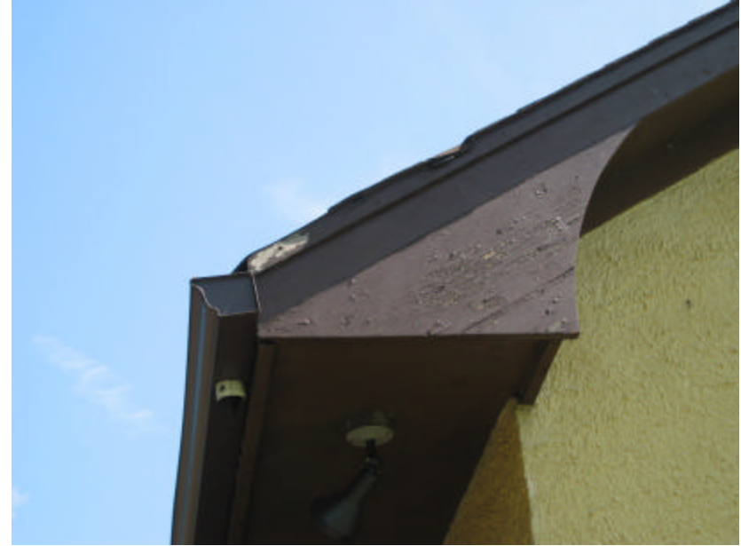
Photo 425 Cracked and peeling paint along the rake of the roof and eaves.
