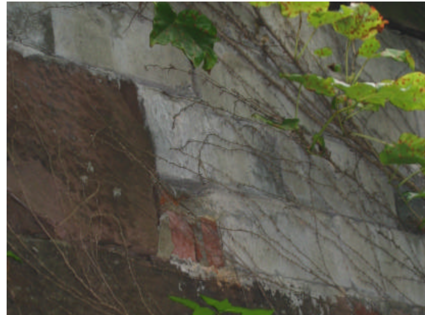
Photo 395 A detail of the remedial patching of the west cheek wall with bricks, concrete blocks and mortar.
