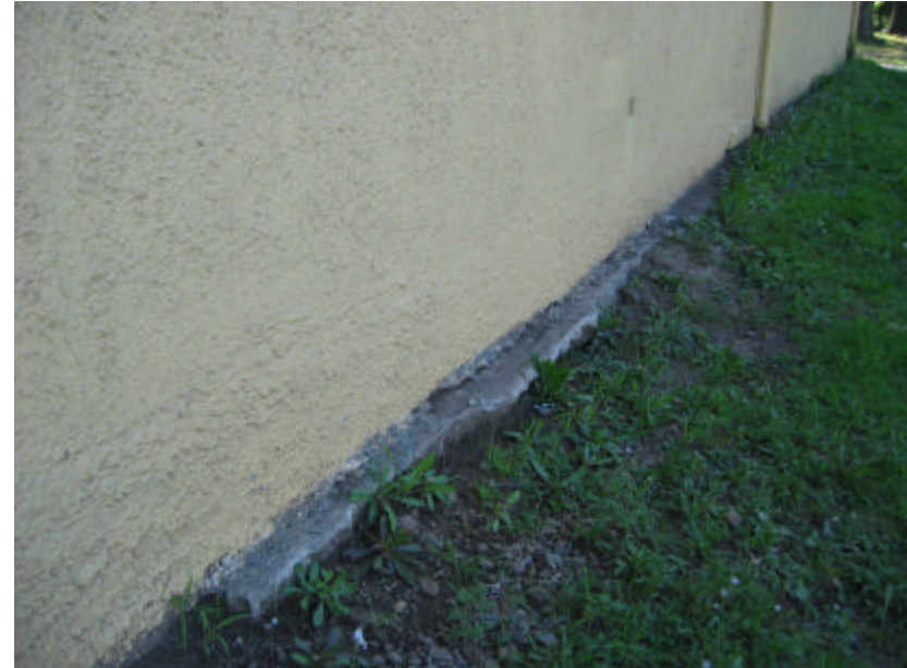
Photo 423 A section of the exposed foundation on the building's north side; note the eroded soil.
