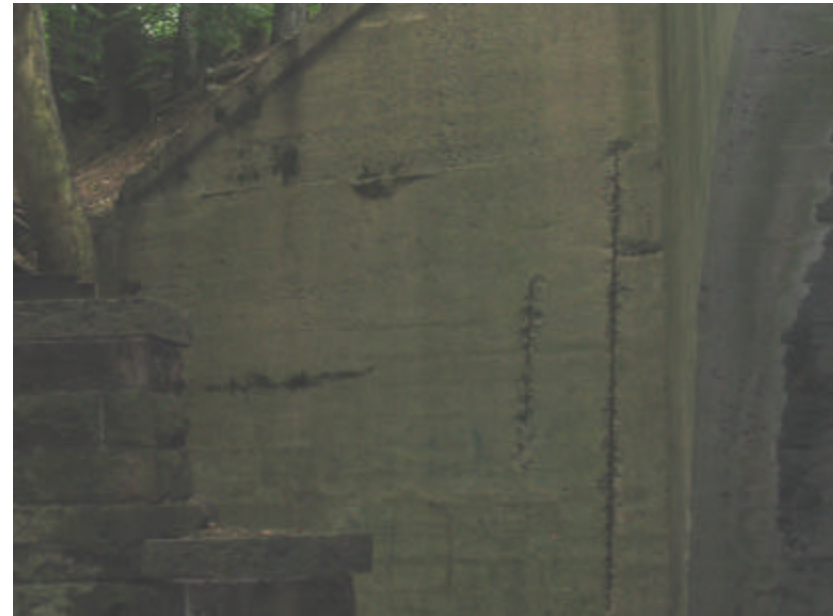
Photo 366 Severe spalling on the southeast wing wall.
