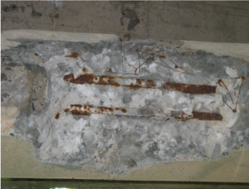
Photo 344 Rusting steel reinforcing exposed by severe spalling underneath the concrete arch.
