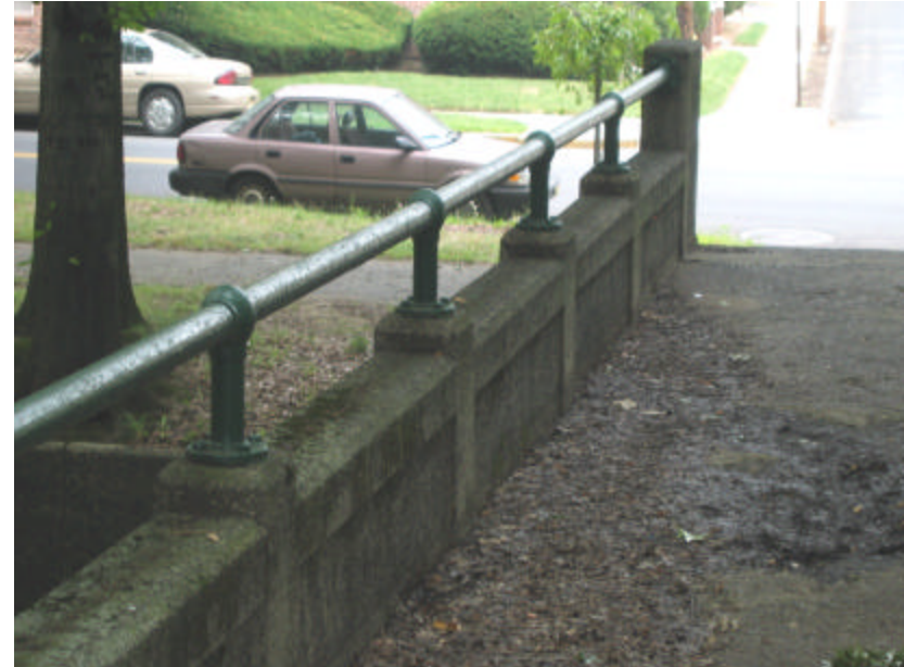
Photo 408 View north towards Mill and Dow Streets, looking over the bridge's deck and railing; note the dirt, leaves and organic growth covering the bridge surfaces.
