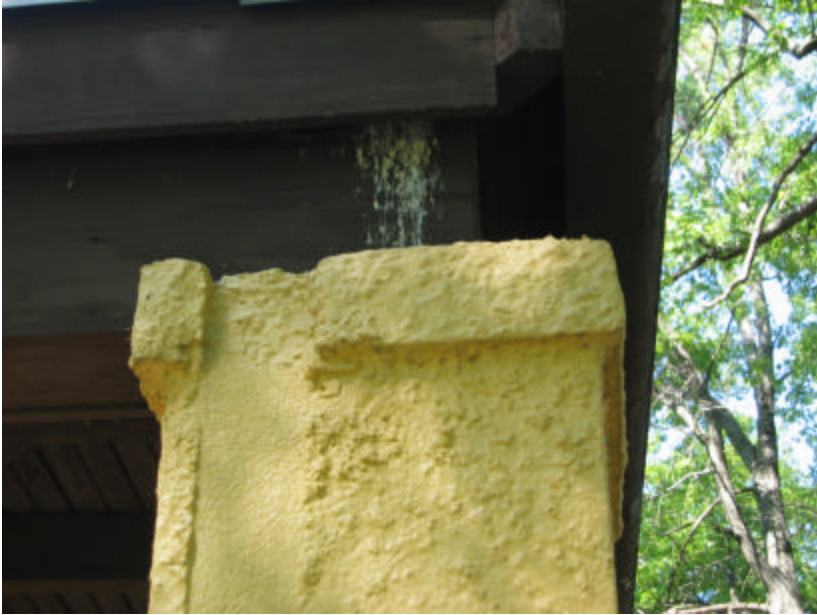
Photo 439 An area of remedial patching on a column.
