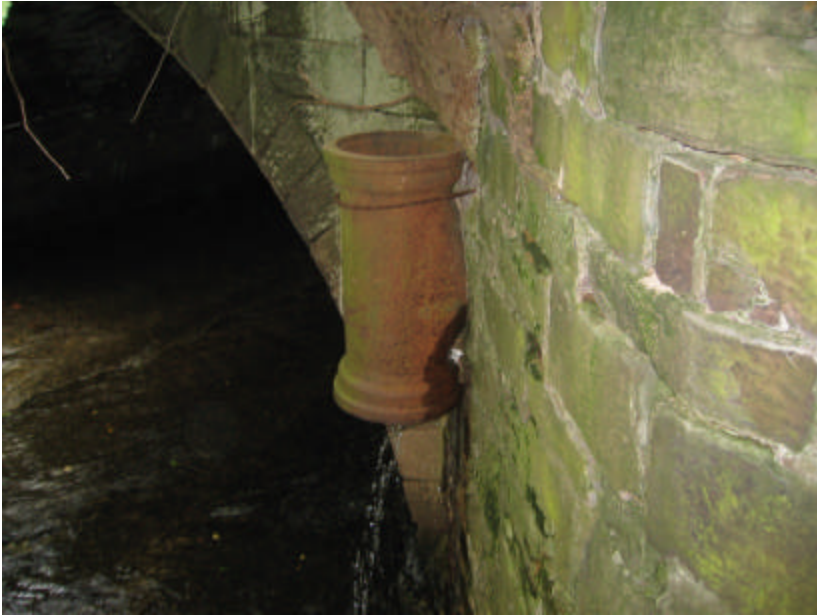
Photo 397 The iron pipe in the wall; note the water coming out the bottom of the pipe.
