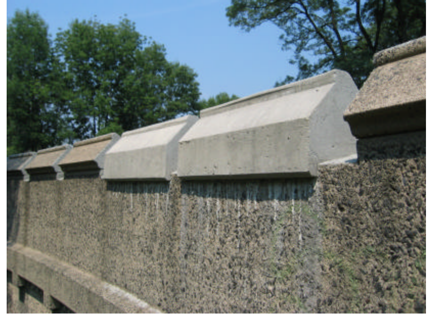
Photo 355 Two new battlements on top of the parapet wall; note that the quality of workmanship and attention to detail is inferior in the newer battlements.
