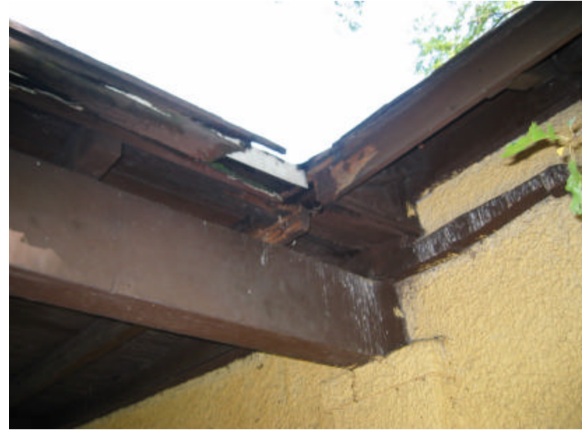
Photo 442 Rotted wood gutter, eaves, sheathing and rafters caused by severe water penetration and lack of maintenance.
