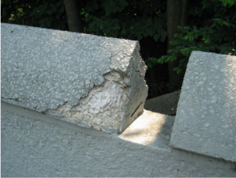
Photo 354 Severely spalled surface of an original coping.
