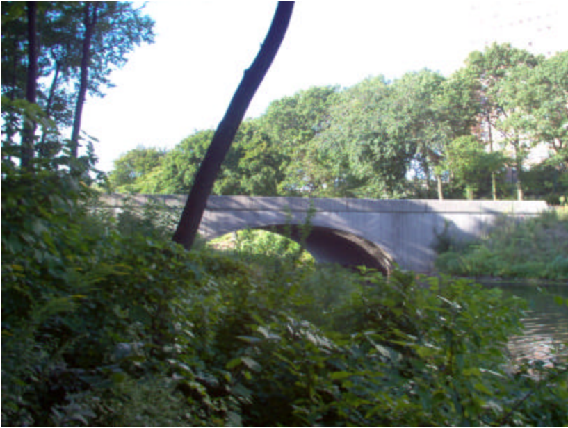
Photo 455 View of South Branch Brook Drive Bridge from the south; note the heavy vegetation growth on the embankment.
