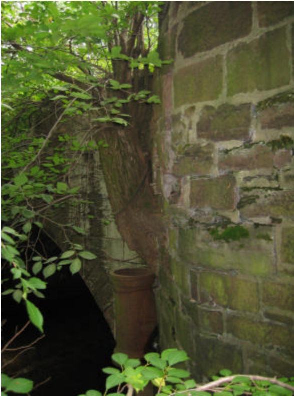
Photo 395 A tree growing out of the south west wing wall; note the pipe piercing the wall below the tree and the significant amounts of vegetation and organic growth.
