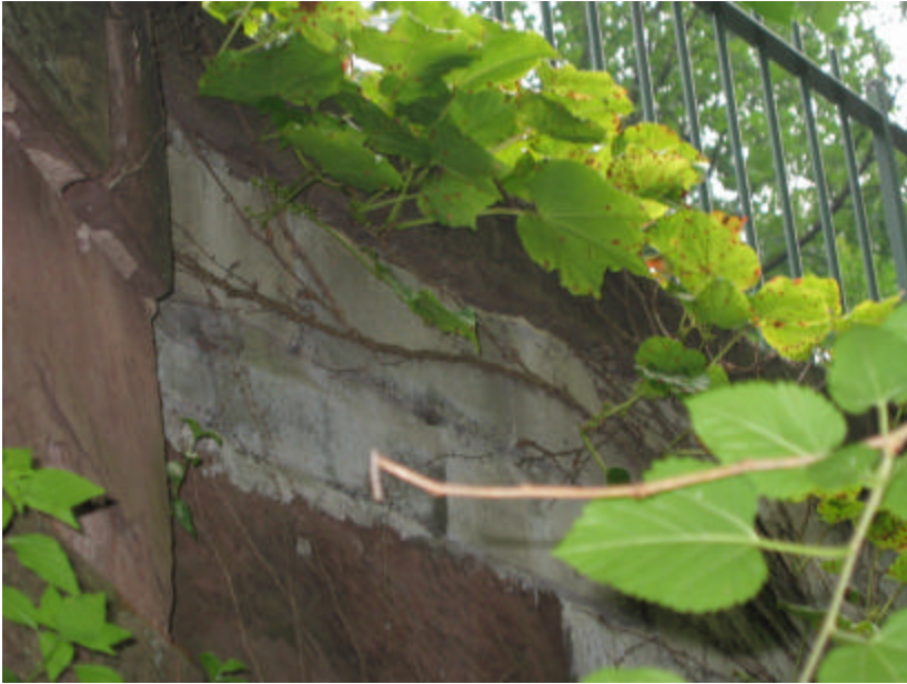
Photo 393 A section of the west cheek wall patched with bricks, concrete blocks and covered with mortar; note the vines covering the surfaces.
