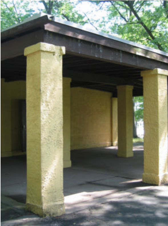
Photo 443 An original wood gutter is visible above the left column; note the staining on the perimeter beam and the damage to the capital.
