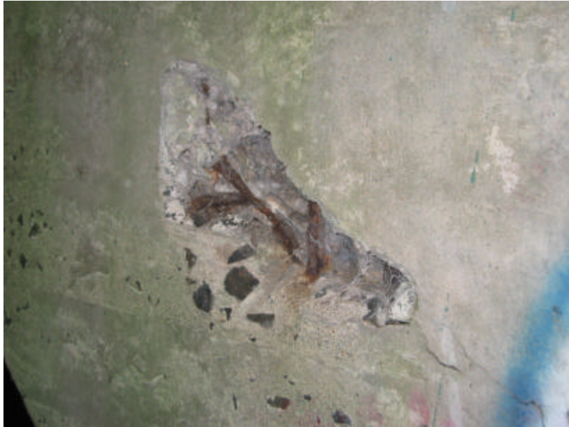
Photo 377 An area of spalling and cracking on the northwest wing wall; note the exposed and rusting steel reinforcing.
