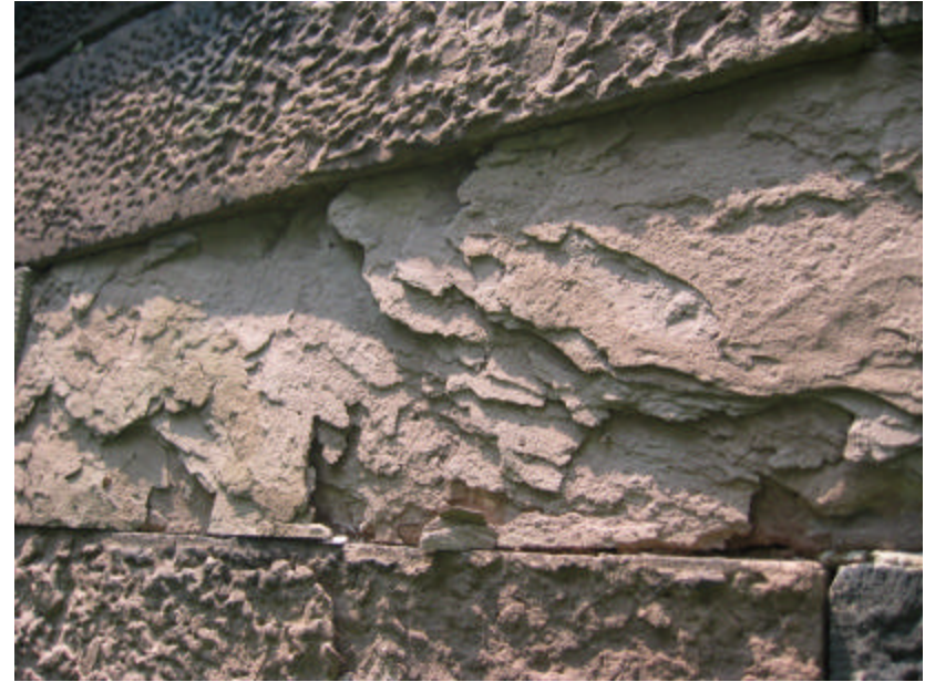
Photo 400 Brownstone delaminating along the bedding plane; note that the mortar has completely eroded from the joints.
