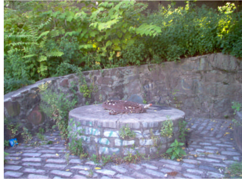
Photo 466 Detail of the northern structure showing displaced grate; note the extensive plant growth.
