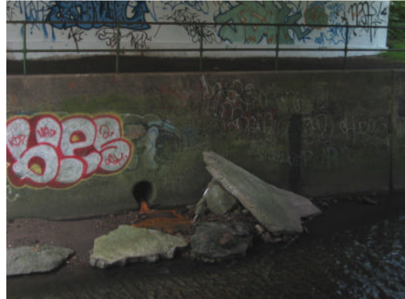
Photo 353 Large sections of concrete in the river below the bridge; note the significant amount of graffiti covering both walls.
