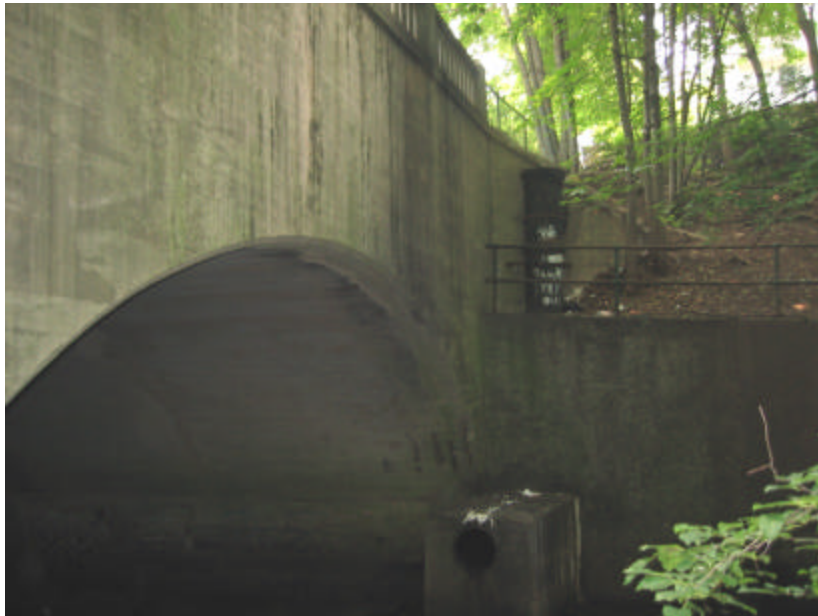
Photo 365 View of the west cheek and wing wall; note the retaining wall, drain pipe and steel pipe railing.
