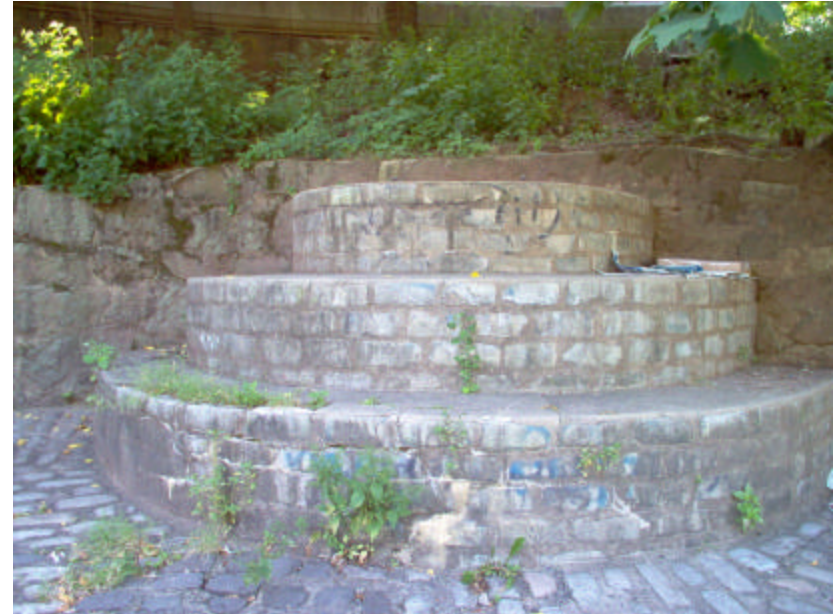
Photo 464 Detail of the center, 3-tiered structure showing some open and failed joints; note the poorly installed, non-matching pavers at patched area. The fieldstone retaining wall rises beyond and encircles the site.
