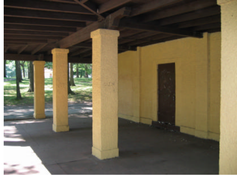
Photo 440 The wood framing of the veranda's roof; note that the columns are in good condition overall.
