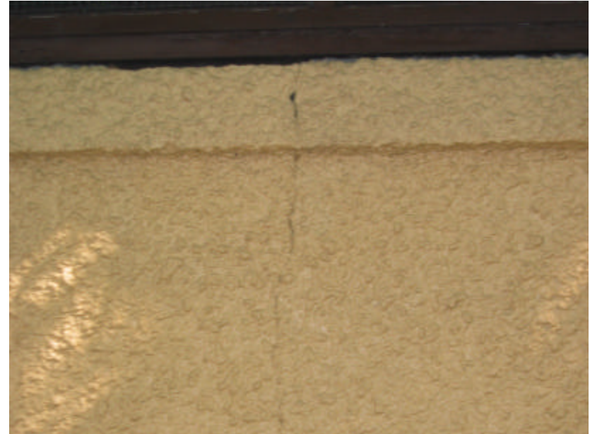
Photo 436 A large vertical crack below one of the windows.
