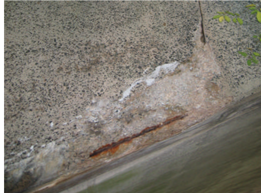
Photo 357 Cracking and spalling where the arch meets the vertical face of the west cheek wall; note the exposed and rusting steel reinforcing.
