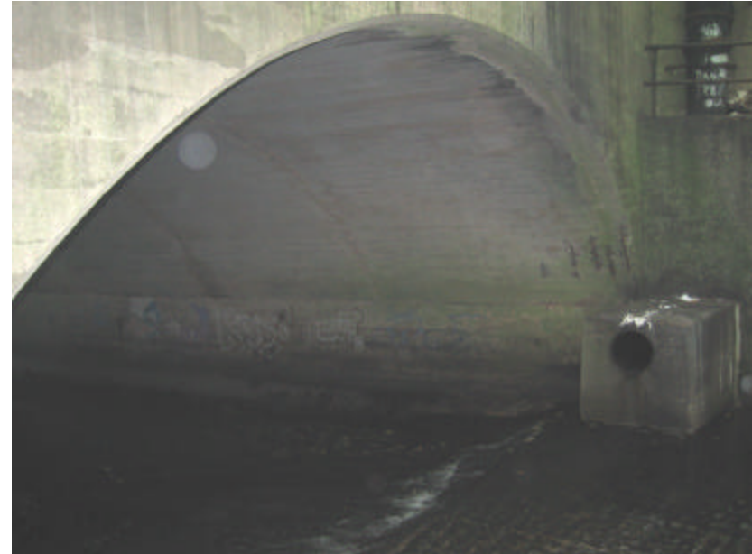
Photo 378 View of the bridge's archway; note the soiling, graffiti and organic growth
