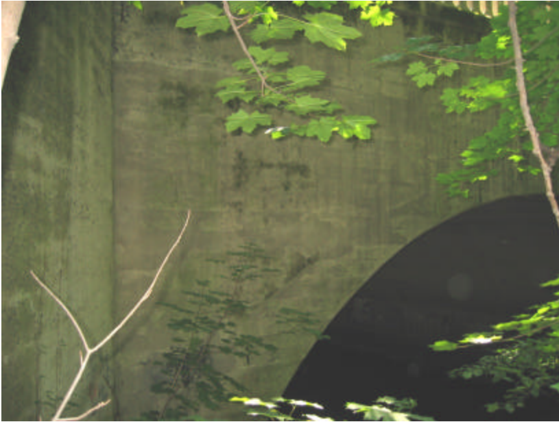
Photo 375 The west cheek and wing walls are in good condition overall; note that there are areas of spalling and organic growth.
