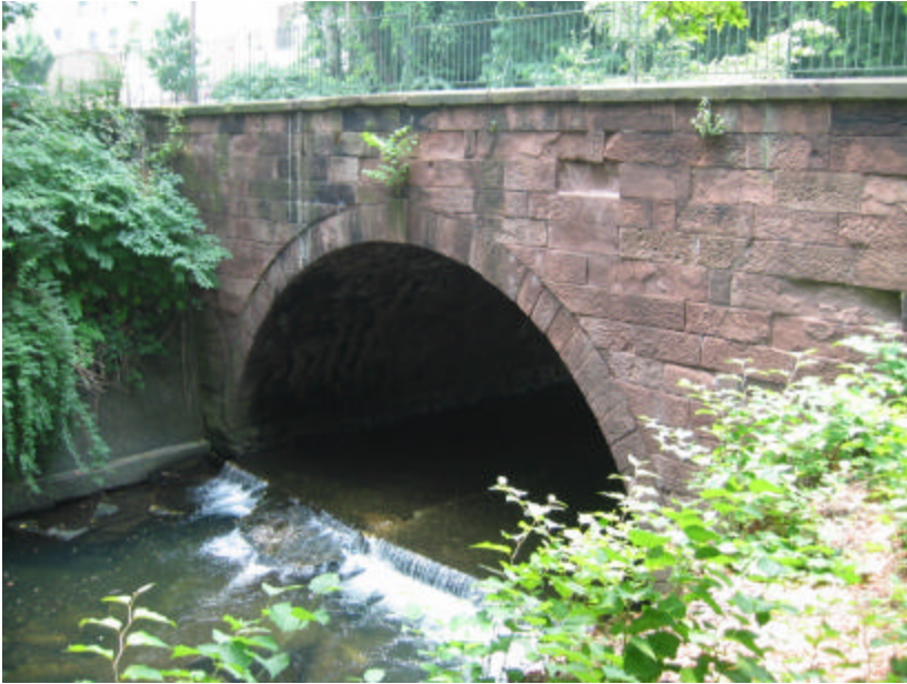
Photo 381 View looking west towards the Summer Avenue Bridge; note the spalled and deteriorated surface of the brownstone.
