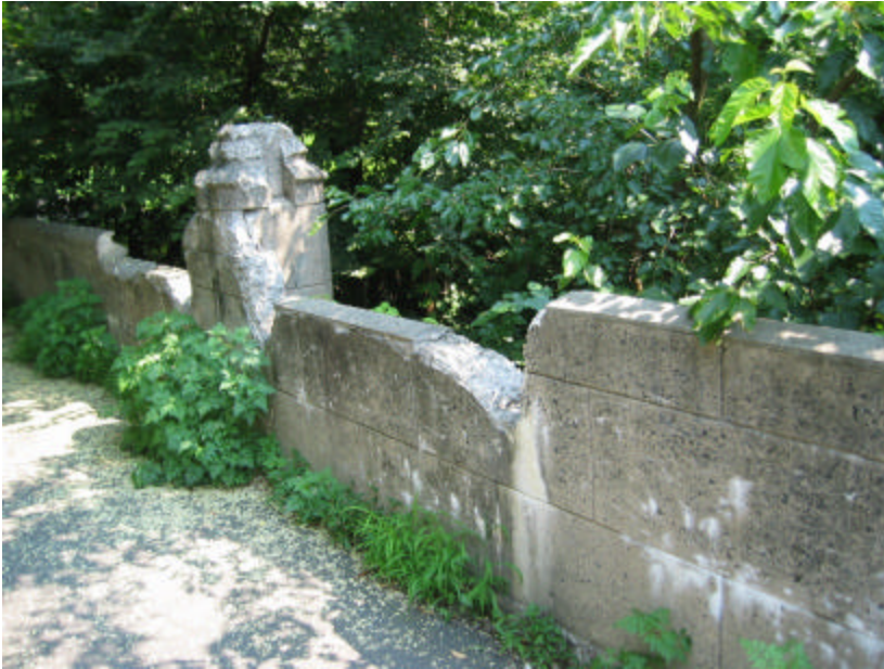
Photo 327 The spalling and cracking parapet walls, copings, and pier caps; note the weeds in the gutter along the base of the wall.
