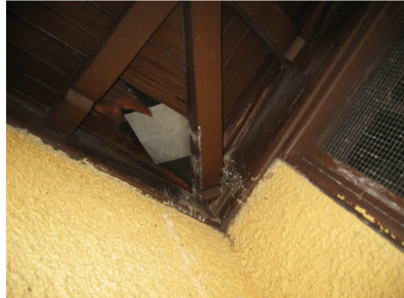
Photo 444 Rotted rafters and sheathing on the west side of the building; note the staining on the wood.
