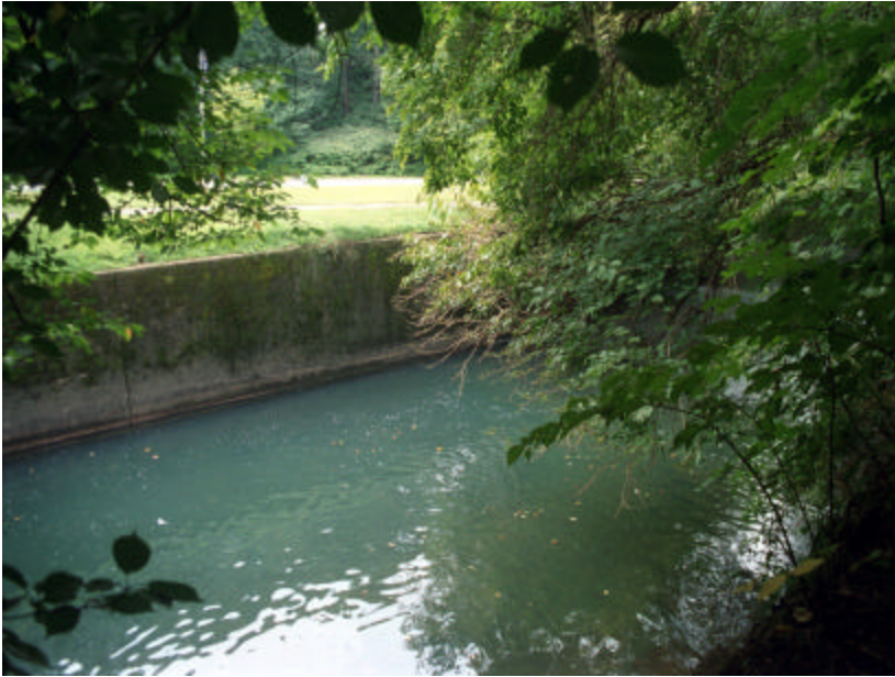
Photo 472 View east of the Franklin Avenue Bridge showing the murky water where the paved channel bed was destroyed.
