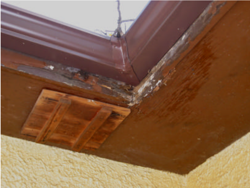
Photo 426 Rotted wood and peeling paint on the eaves; note that a section of the soffit has been patched with plywood.
