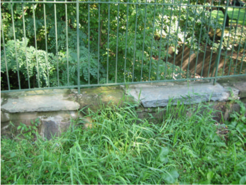
Photo 391 Bluestone is being used instead of brownstone as material for coping on top of the south end of the west wing wall.
