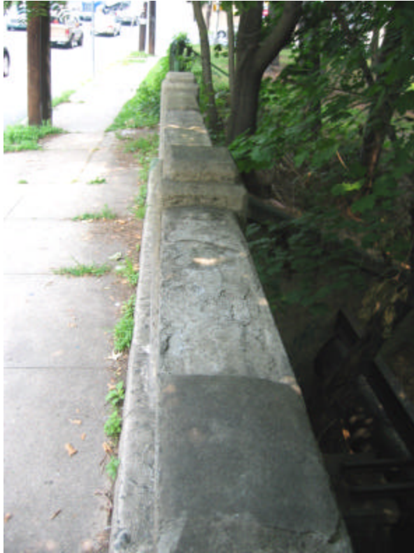
Photo 373 An area of severe spalling and missing concrete on top of the east railing; note the grass and weeds growing from cracks in the sidewalk.
