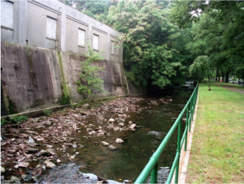
Photo 488 View looking west toward the Summer Avenue Bridge, where the typical south revetment vertical wall is interrupted by the large, battered retaining wall.
