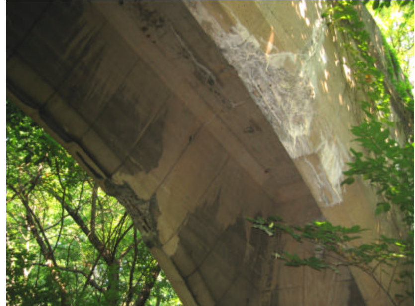
Photo 343 An area of extreme spalling and cracking; note the exposed steel reinforcing, de-icing and other soluble salts and mineral deposits.
