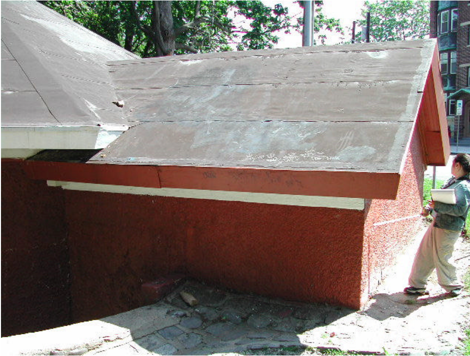
Photo 454 Detail of Octagon Field House from the southwest showing non-original roll roofing and non-original plywood cladding on cornice.
