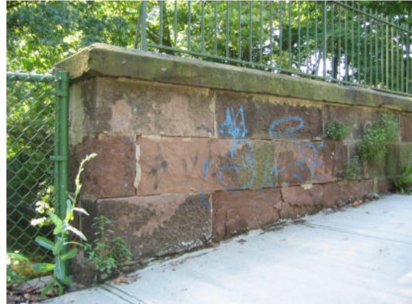
Photo 389 The north end of the east parapet wall; note the change in grade from left to right. Also note the severely spalled brownstone surfaces and graffiti.
