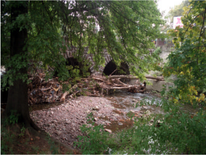
Photo 492 Debris build-up along the commercial site walls immediately to the west.
