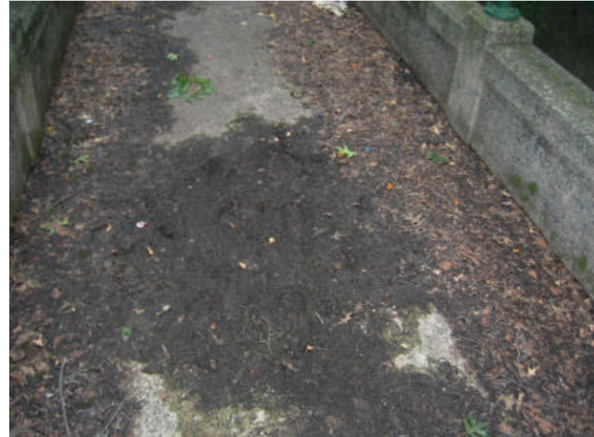
Photo 412 Leaves and mud covering the bridge's deck; note that this debris covers a large area of spalling concrete.
