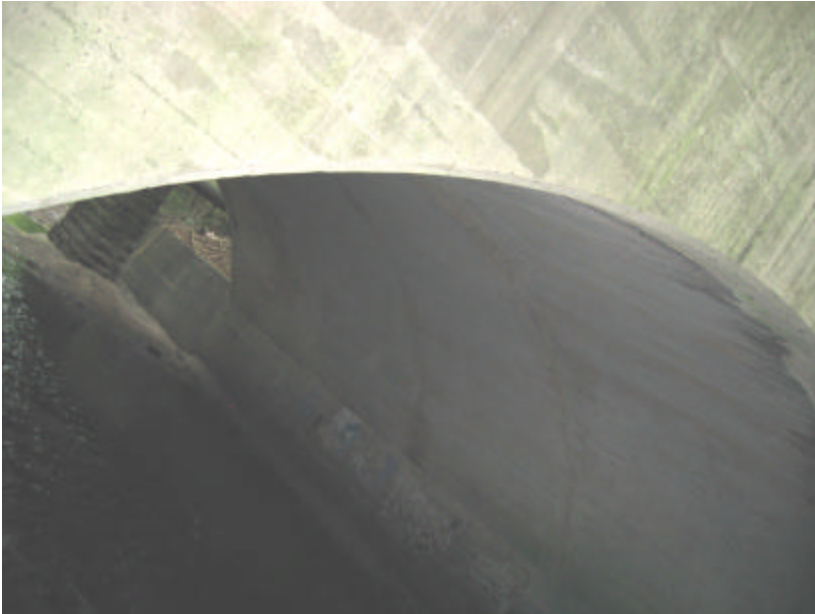
Photo 379 View of the bridge's west vertical face and archway; note the soiling, graffiti and organic growth.
