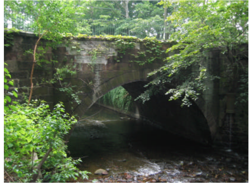
Photo 382 View looking east towards the Summer Avenue Bridge; note the significant amount of plant growth and the area of brick patching covered with white mortar.
