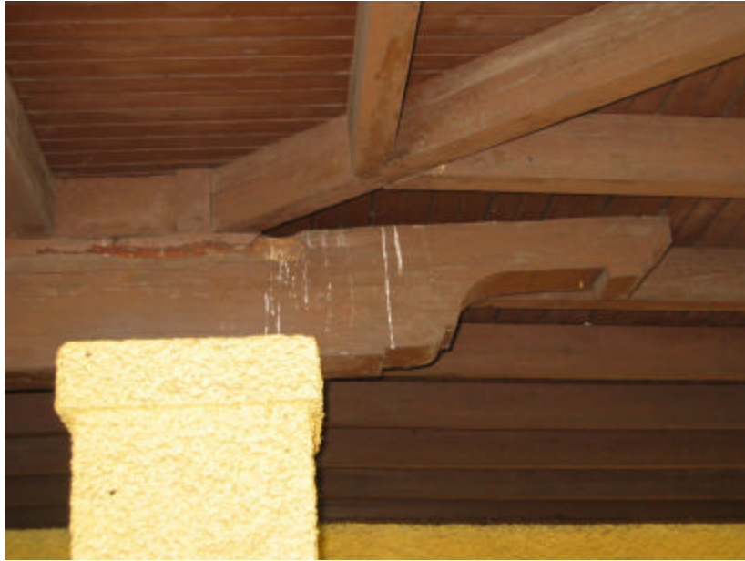
Photo 433 A beam spanning between two of the square columns in the center of the veranda; note that a section of the beam is cracked and rotted.
