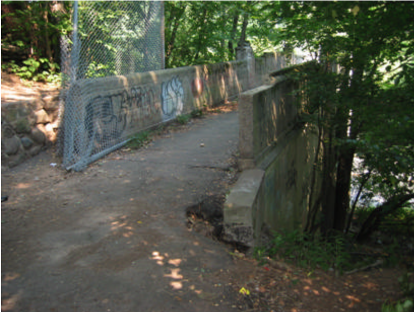
Photo 332 View towards the south end of the bridge; note the severe erosion to the right of the photo evidencing damage by water runoff.
