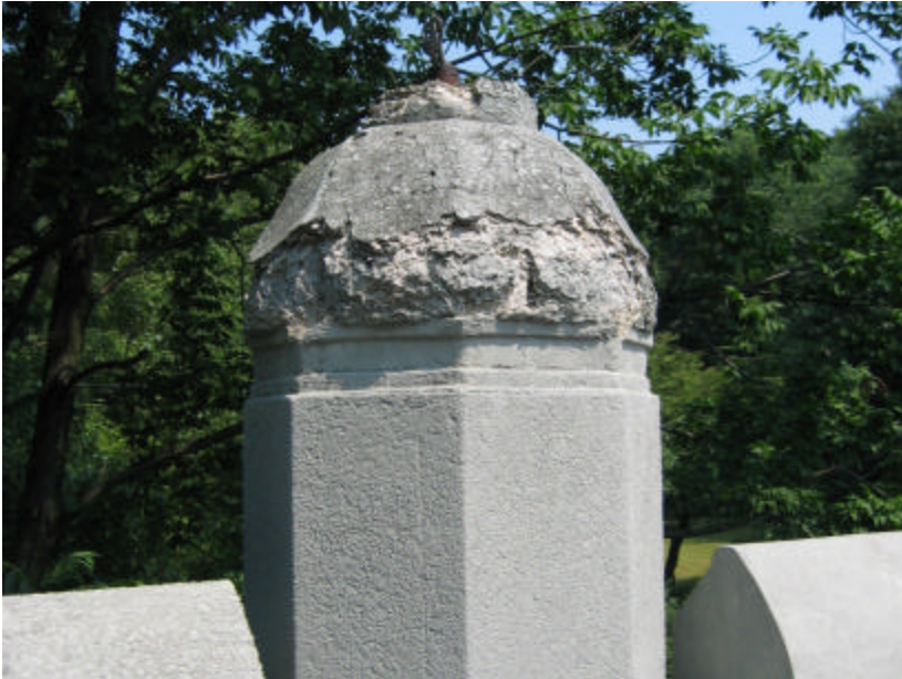
Photo 352 A lantern base that surmounts one of the buttresses; note the severe spalling.
