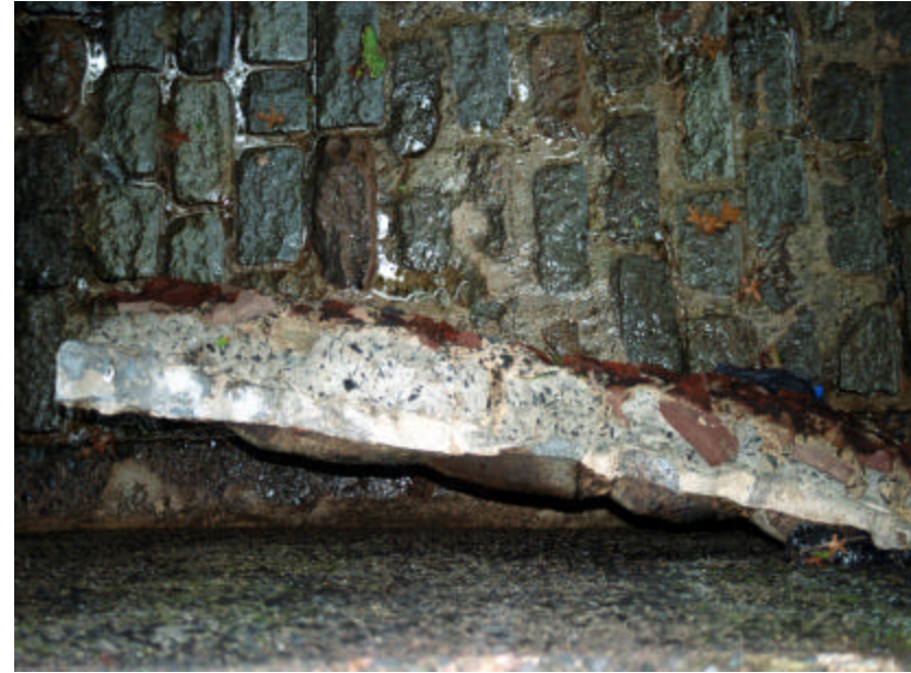
Photo 479 Detail of cross section of dislodged channel paving showing concrete base with embedded brownstone from the river channel bed and granite pavers embedded in concrete mortar.
