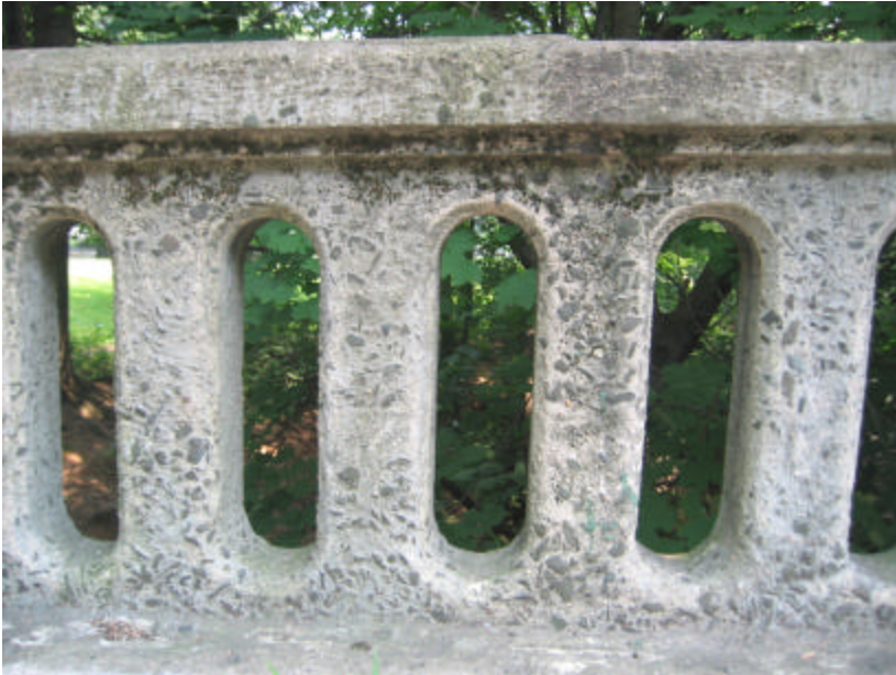
Photo 371 Oval openings on the east side of the bridge showing the weathered surface; note the organic growth directly below the top of the railing.
