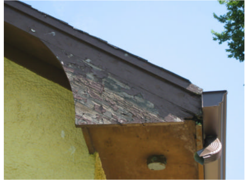
Photo 417 Cracked and peeling paint on the rake and soffits of the roof; note that the gutter's downspout is missing.
