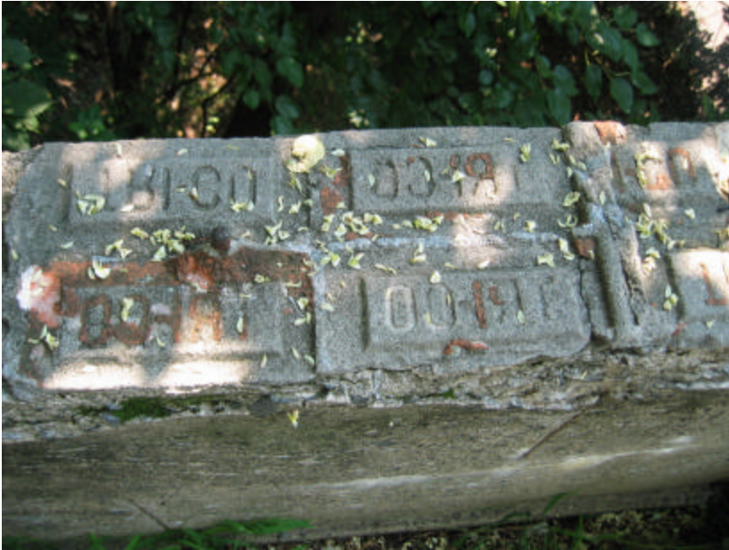
Photo 342 Detail looking down at the top of a parapet wall, showing remedial patching by replacement bricks.
