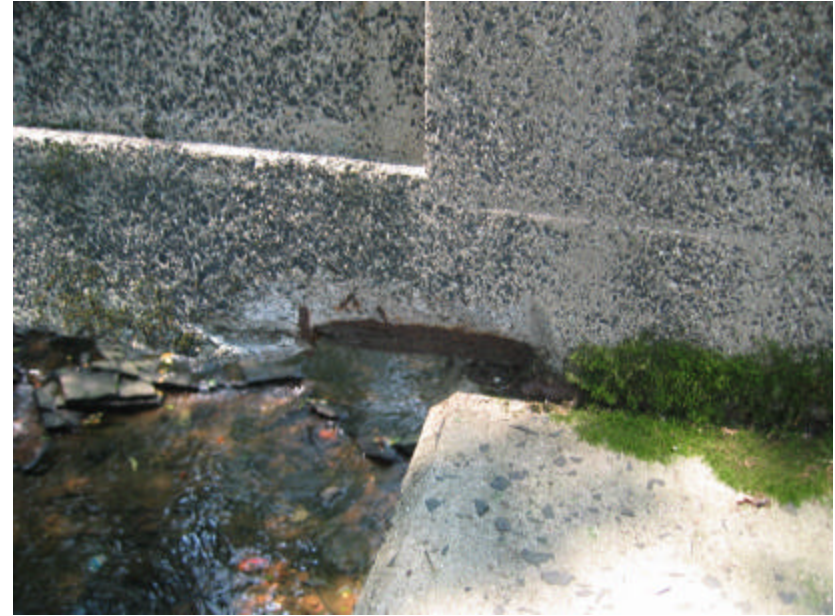
Photo 410 A detail of the spalling and organic growth at the north end of the bridge.
