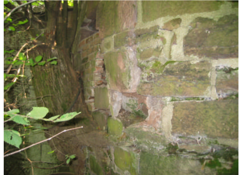
Photo 396 The tree and its roots have caused significant damage to the wall; note the cracked and displaced masonry and the remedial brick patching.
