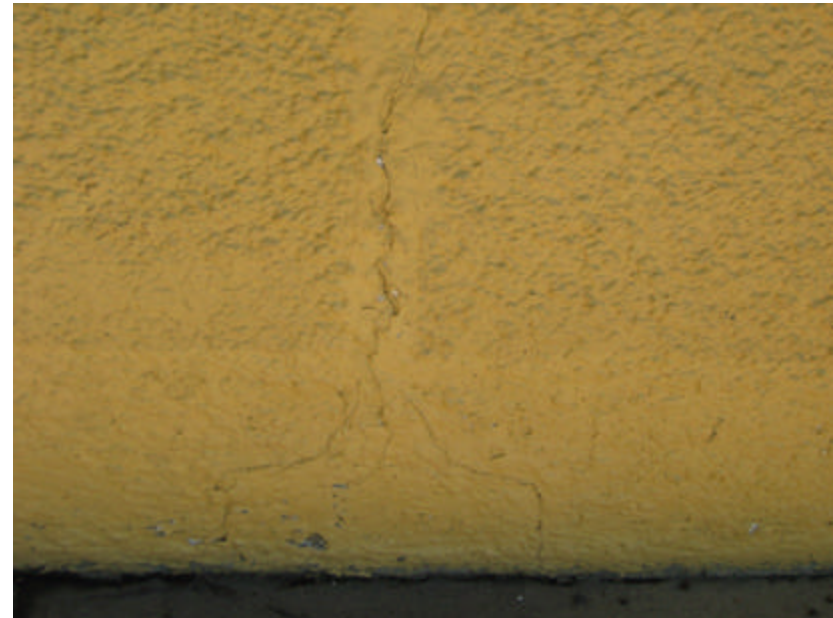
Photo 415 Cracked stucco on the southwest wall; note that the crack has been patched and painted.
