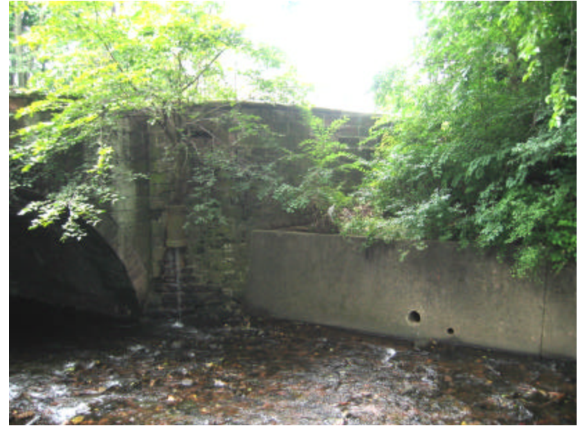
Photo 384 View southeast towards the bridge; note the significant amount of plant growth, including a tree growing from the wing wall.
