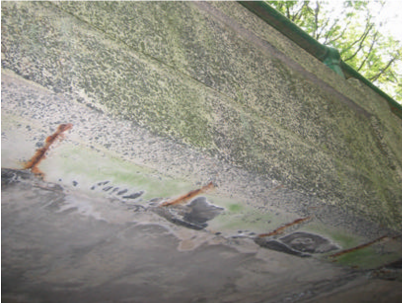
Photo 411 View looking up at the bottom of the bridge; note the areas of rust and water staining.
