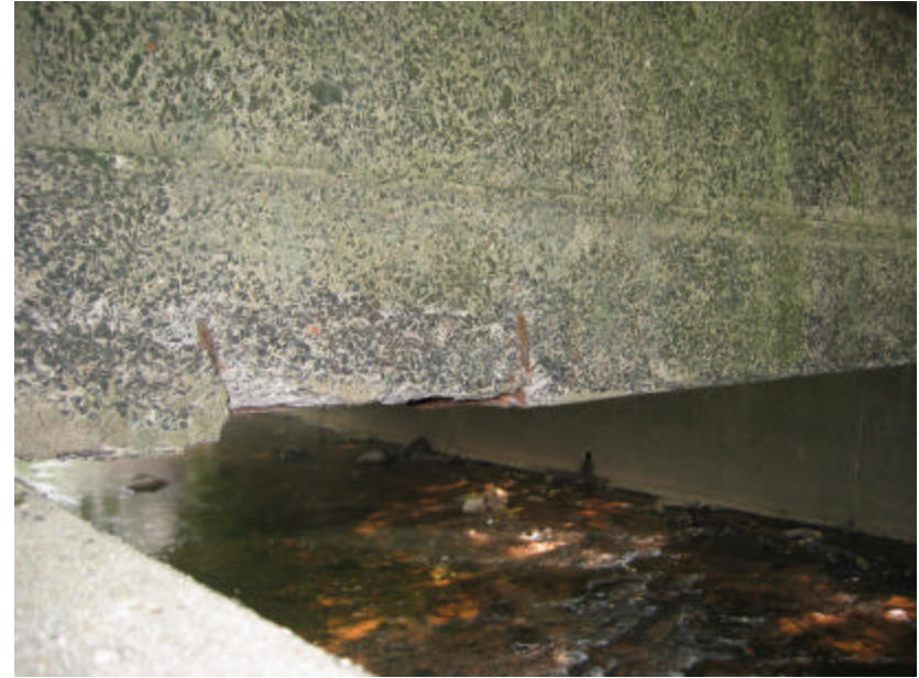
Photo 406 An area of spalling on the base of the bridge.
