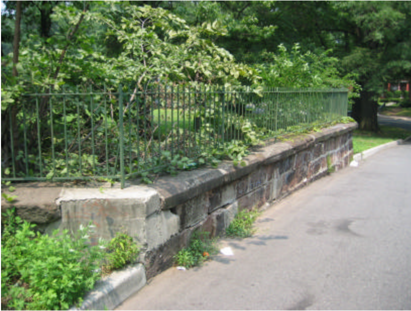
Photo 383 The parapet wall and metal fence atop the cheek wall; note the poor condition of the brownstone and the section of concrete patching.
