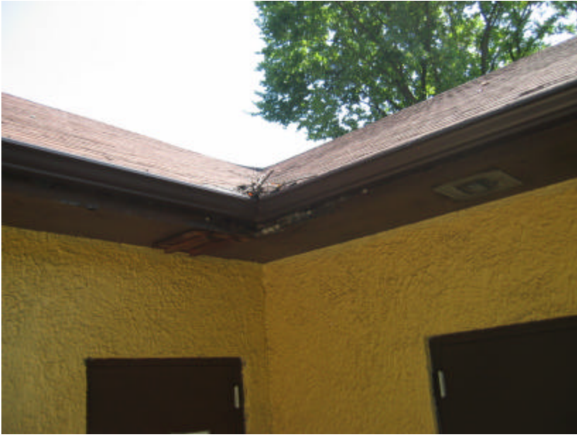
Photo 416 Rotting and cracked plywood soffit caused by water damage because of debris collecting in the gutter.
