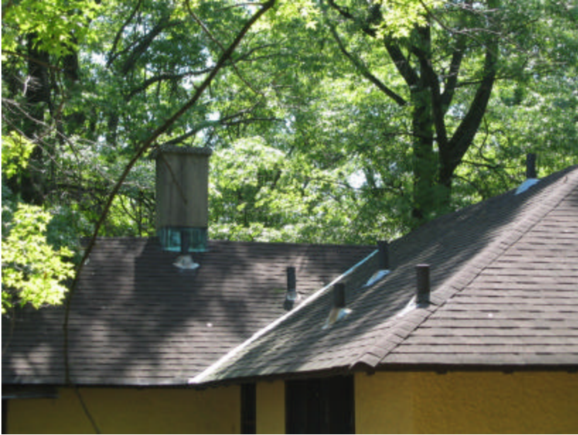
Photo 445 The asphalt-shingled hip roof; note all the steel pipe penetration and the masonry chimney.
