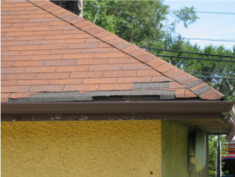
Photo 428 Some missing asphalt shingles on the west side of the building; note that the shingles hang down into the gutter.
