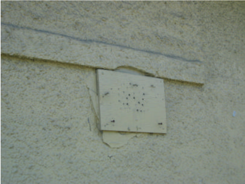
Photo 422 Plywood covering a hole in the wall below one of the original windows.
