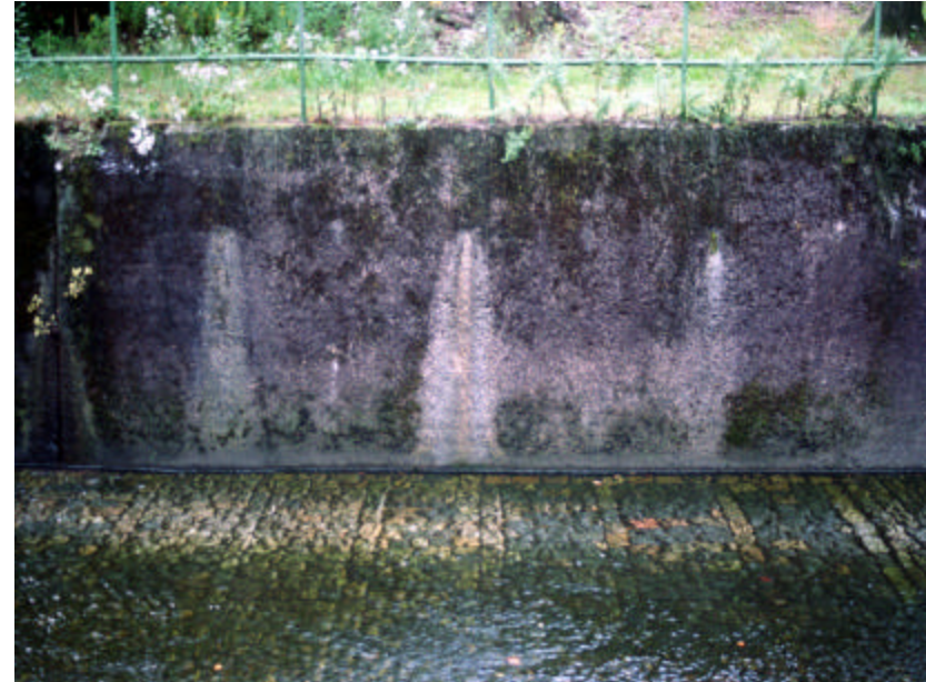
Photo 475 Detail of South revetment and stone-paved channel bed immediately west of the North Branch Brook Drive Bridge; note the moss growth, erosion and the modest spalling of concrete walls.
