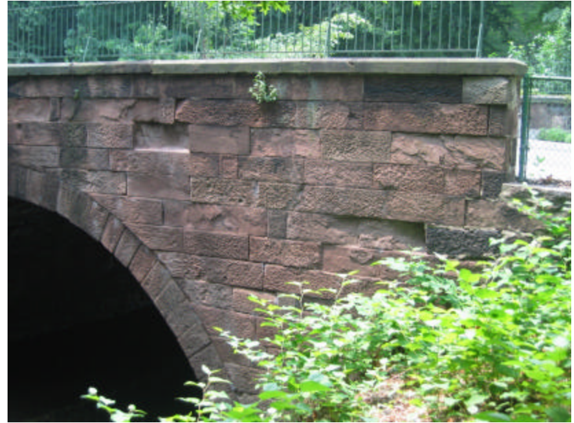
Photo 398 The east cheek and parapet wall; note the fence on top of the copingstones.
