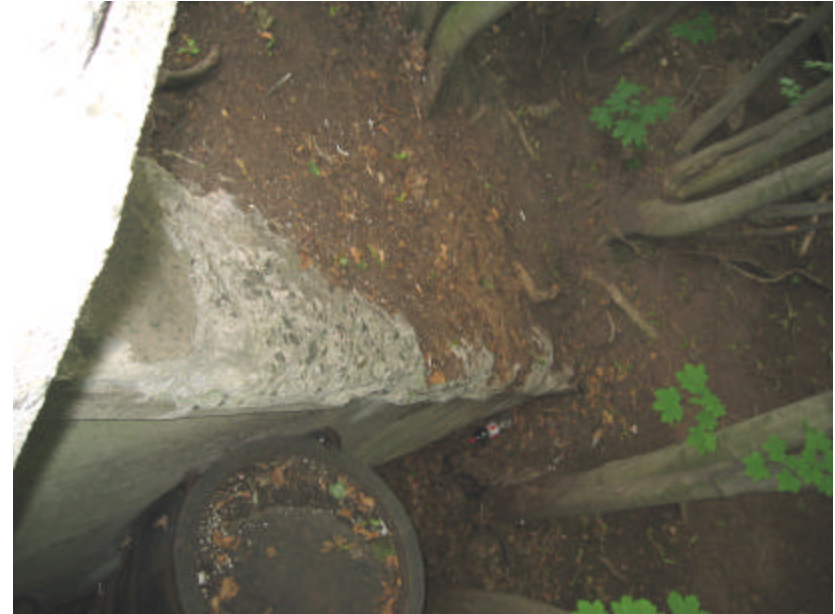
Photo 374 Severe spalling on the southwest wing wall; note the erosion around the site and the steel barrels at the bottom of the photo.
