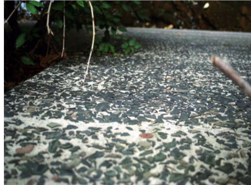
Photo 469 Detail of exposed aggregate on the vertical faces of the revetment wall.
