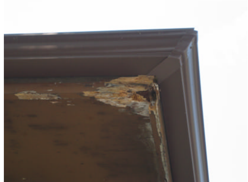
Photo 427 Rotted wood and peeling paint on the soffit; note that the water damage on the soffits of this building usually occurs at the corners.
