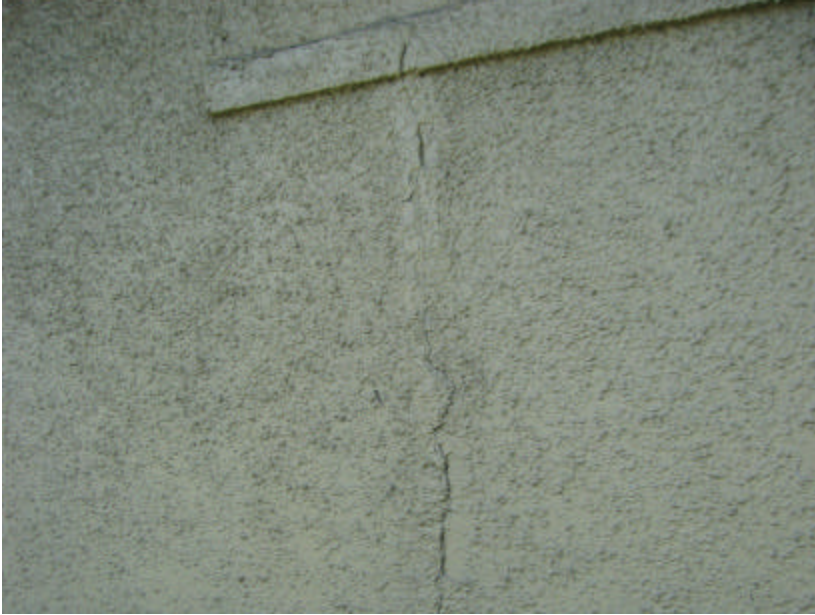
Photo 424 Cracking on the north wall that has been poorly patched and painted.
