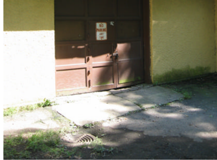
Photo 446 The wood garage door at the rear of the building; note that the concrete apron is severely cracked.
