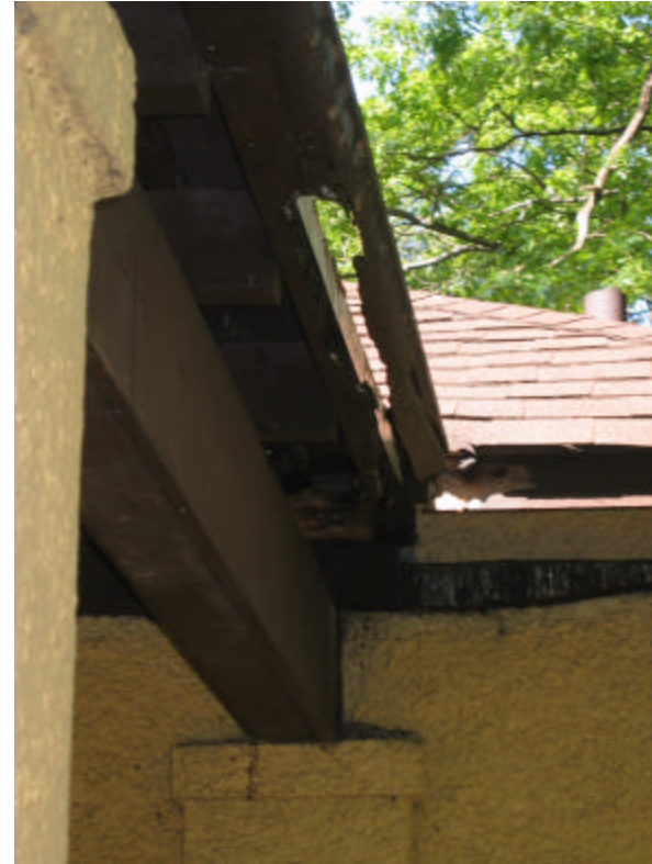
Photo 432 One of the severely rotted wood gutters on the east side of the veranda; note the water damage to the sheathing.
