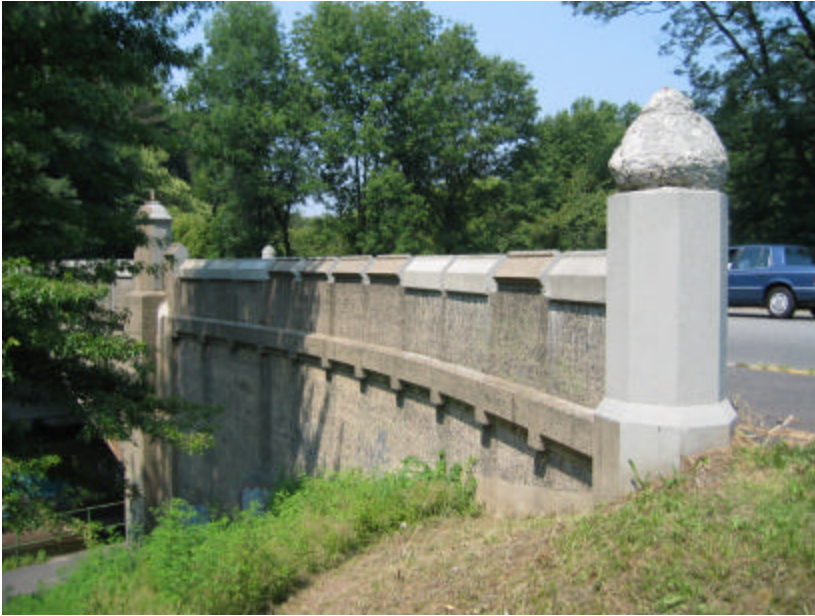
Photo 350 The wing and parapet wall on the north side of the bridge; note that the top of the post has severely spalled and many of the battlements surmounting the parapet walls have been replaced.
