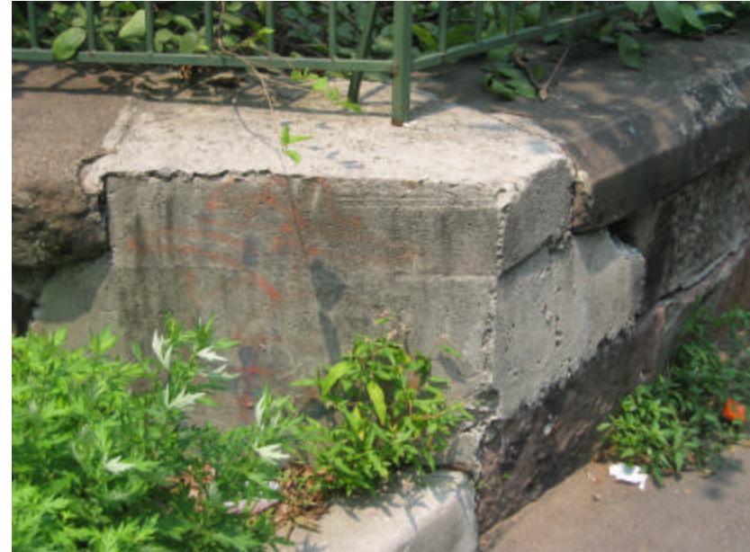
Photo 390 A large section of the parapet wall patched with concrete.
