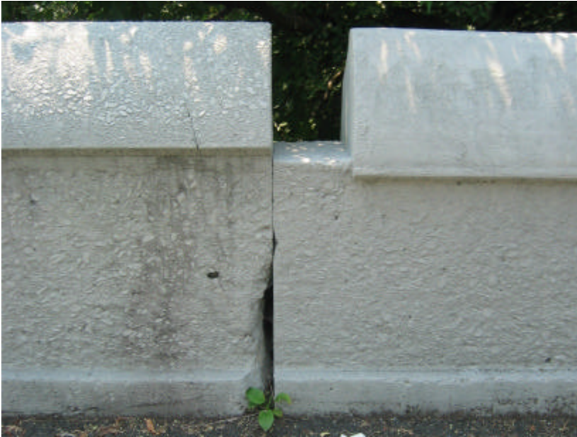
Photo 360 This crack is directly across the street in the same location.
