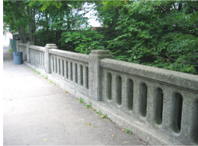
Photo 368 The west parapet railing; note that it is in good condition overall but it has suffered weathering, which has exposed the concrete aggregate.
