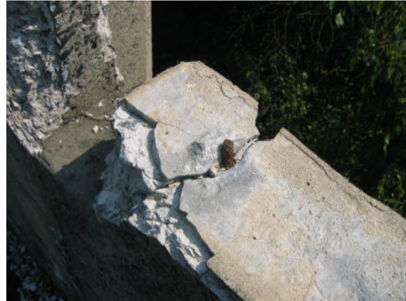
Photo 341 Severe cracking and spalling around a piece of exposed, rusting steel reinforcing.
