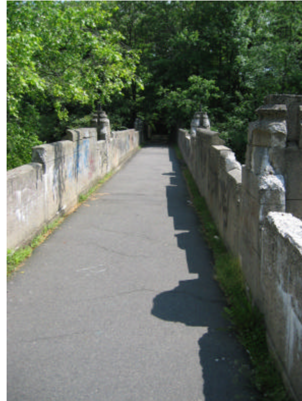
Photo 329 The paved asphalt pathway over the bridge; note the extremely poor condition of the parapet walls, copings, pier caps and lantern bases. Also note that weeds and organic debris clog the gutters on both sides of the bridge.
