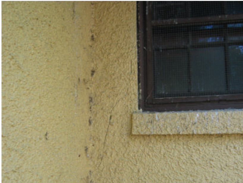
Photo 437 A crack that runs parallel to a window; note the staining on the stucco's surface.
