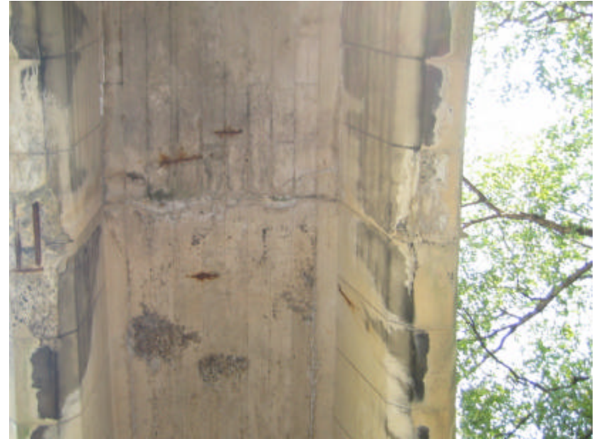
Photo 345 This spalling and cracking extends underneath the entire bridge; note the areas of soiling, staining and exposed steel reinforcing.
