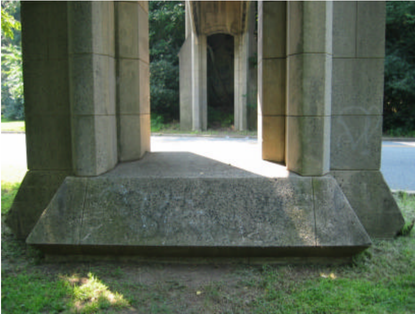
Photo 325 The massive foundation caps and footings supporting the twin piers; note the graffiti and organic growth on the surfaces.
