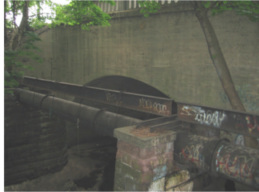
Photo 376 The east cheek and wing walls are in good condition overall; note the pipe crossing the Second River directly east of the bridge.
