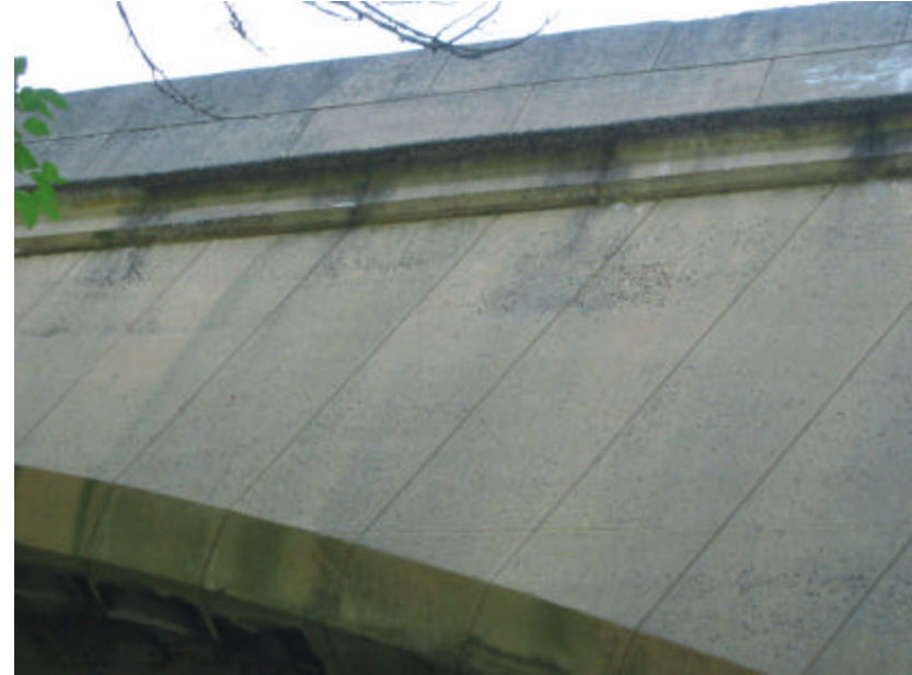
Photo 326 The bridge's scored concrete surfaces simulating stonework; note that this section of the bridge is in fair condition.
