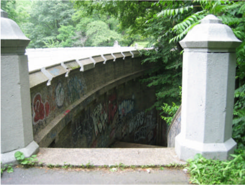
Photo 364 The parapet and wing wall adjacent to the staircase are covered with graffiti.
