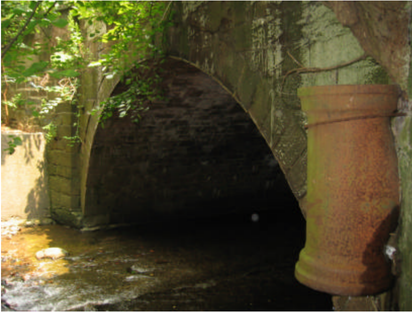
Photo 401 View of the archway; note the organic growth and efflorescence covering the surfaces.
