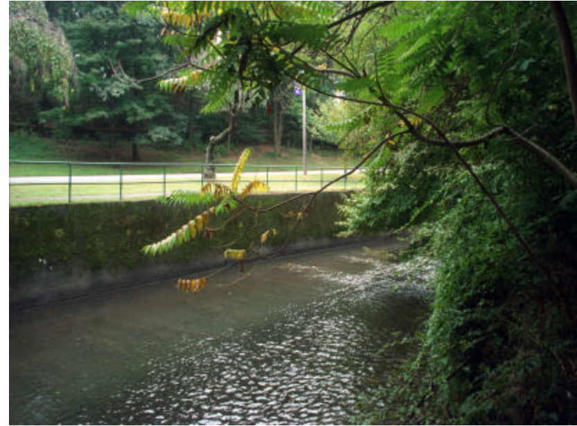
Photo 471 View west of The Erie Railroad Bridge, looking to the south revetment wall and with North Branch Brook Drive beyond, showing continuous and massive moss growth on channel walls; note the pattern at the channel bed created by the granite pavers.
