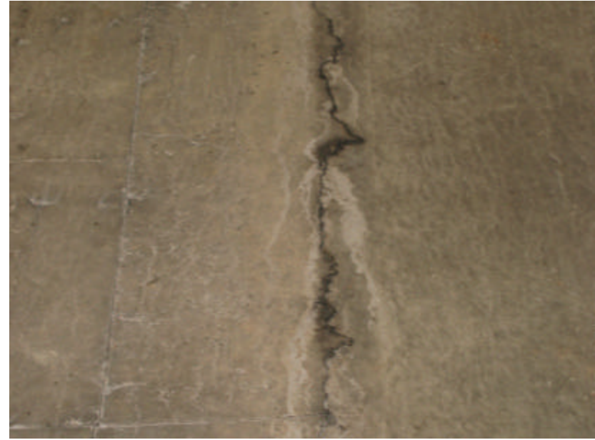
Photo 361 Cracking on the surface of the arch; note the soiling and water staining.
