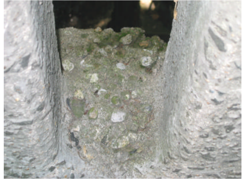
Photo 370 An area of remedial concrete patching at the base of an oval opening on the east side of the bridge.
