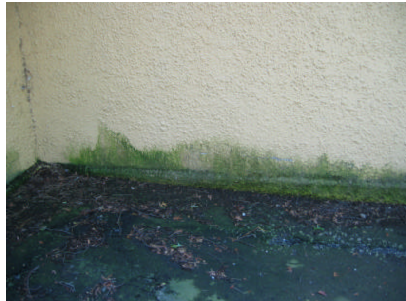
Photo 438 Organic growth and debris at the base of a wall; note that the site has poor drainage in many locations.
