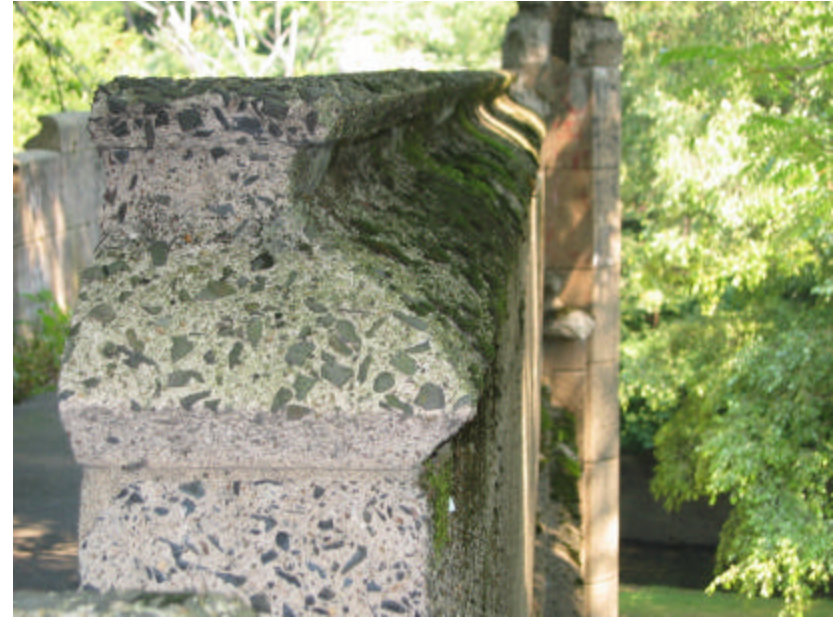
Photo 337 The finished end of an original piece of coping; note that years of weathering have eroded the surface, exposing the aggregate.
