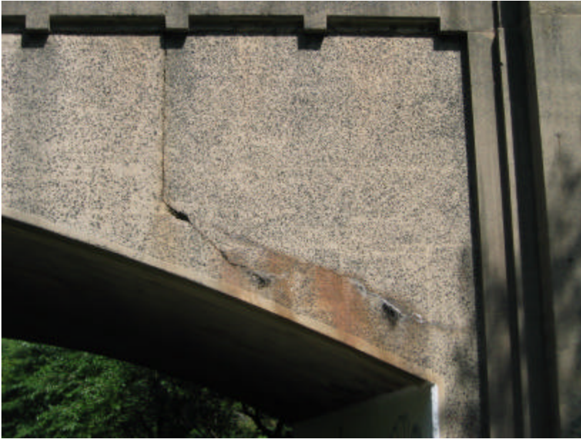
Photo 356 Cracking along the cold joint in the parapet wall continues through the cheek wall; note the differences in the concrete finishes between the wall and the buttress.
