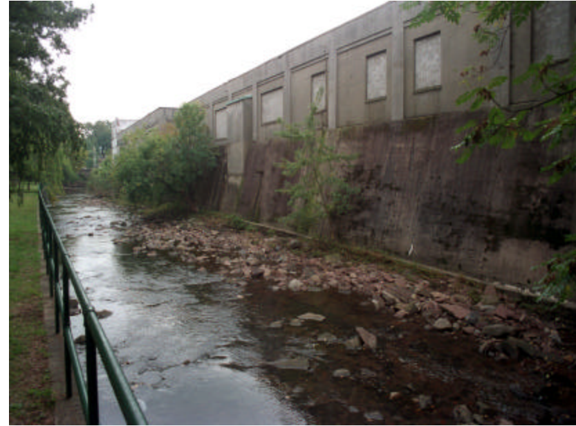
Photo 489 Detail of the south revetment retaining wall showing spalled concrete and significant natural debris accumulation.
