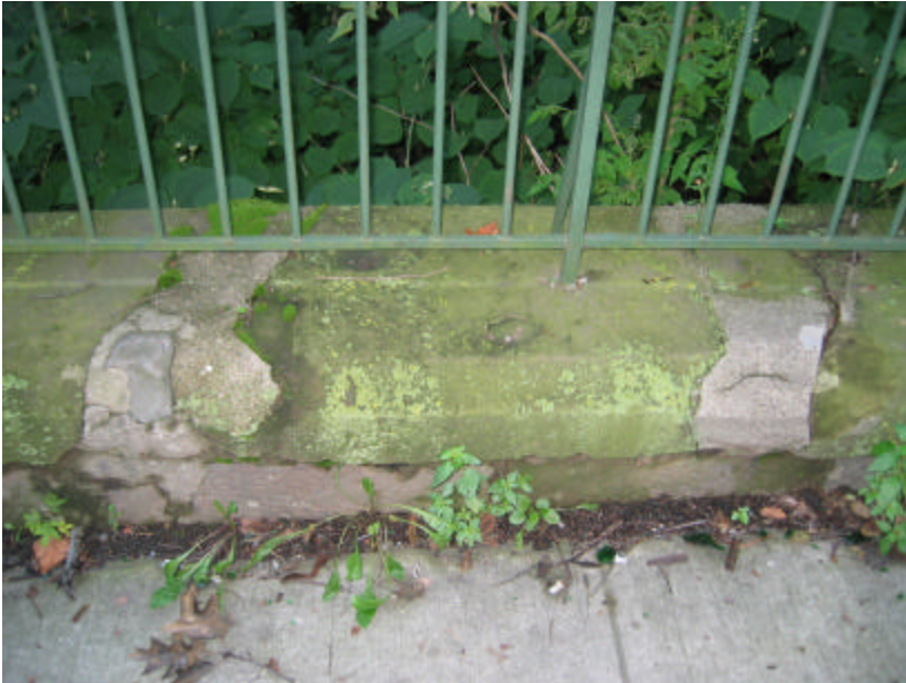
Photo 389 Remedial patching of copingstones with concrete; note that organic growth has discolored the stone surface, turning it green.
