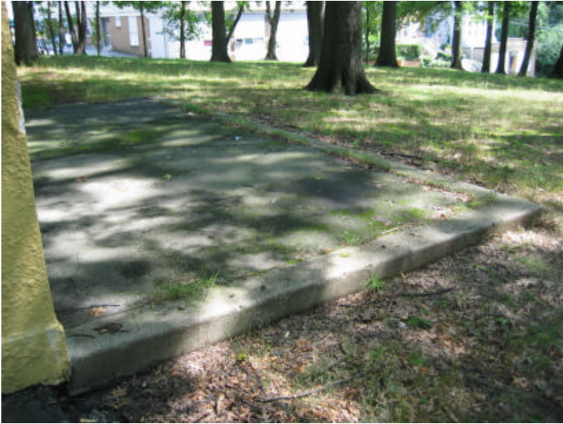
Photo 447 One of the original sand courts that has been covered with asphalt; note that the paving is now cracked and buckled.
