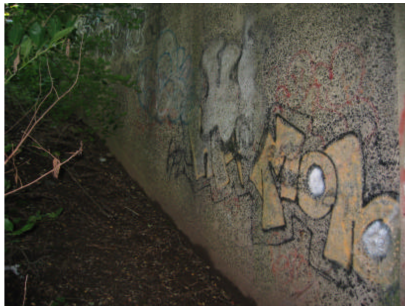
Photo 363 The north wing wall on the east side of the bridge is covered with graffiti.
