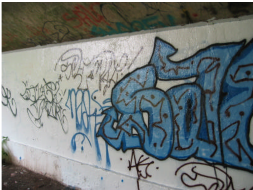
Photo 362 A painted wall covered with graffiti on the south side of the bridge.
