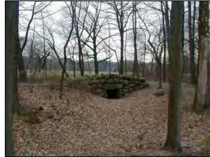
Dry streambed in the vicinity of Brookside Meadow Bridge (looking north with the North Playfield visible in the background through the trees).
